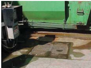
A drain adjacent to a trash compactor is connected to the sanitary sewer system. A concrete berm surrounding the trash storage area hydraulically isolates stormwater runoff in this area from the rest of the site.
