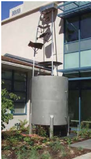
A cistern at Mills College in Oakland, CA is a stormwater BMP and a design element. Photo: Ingrid Severson
