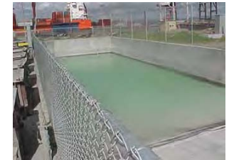
Rainwater harvesting is a volume-based BMP that can be used to collect water for various types of industrial operations, resulting in reduced utility costs.
