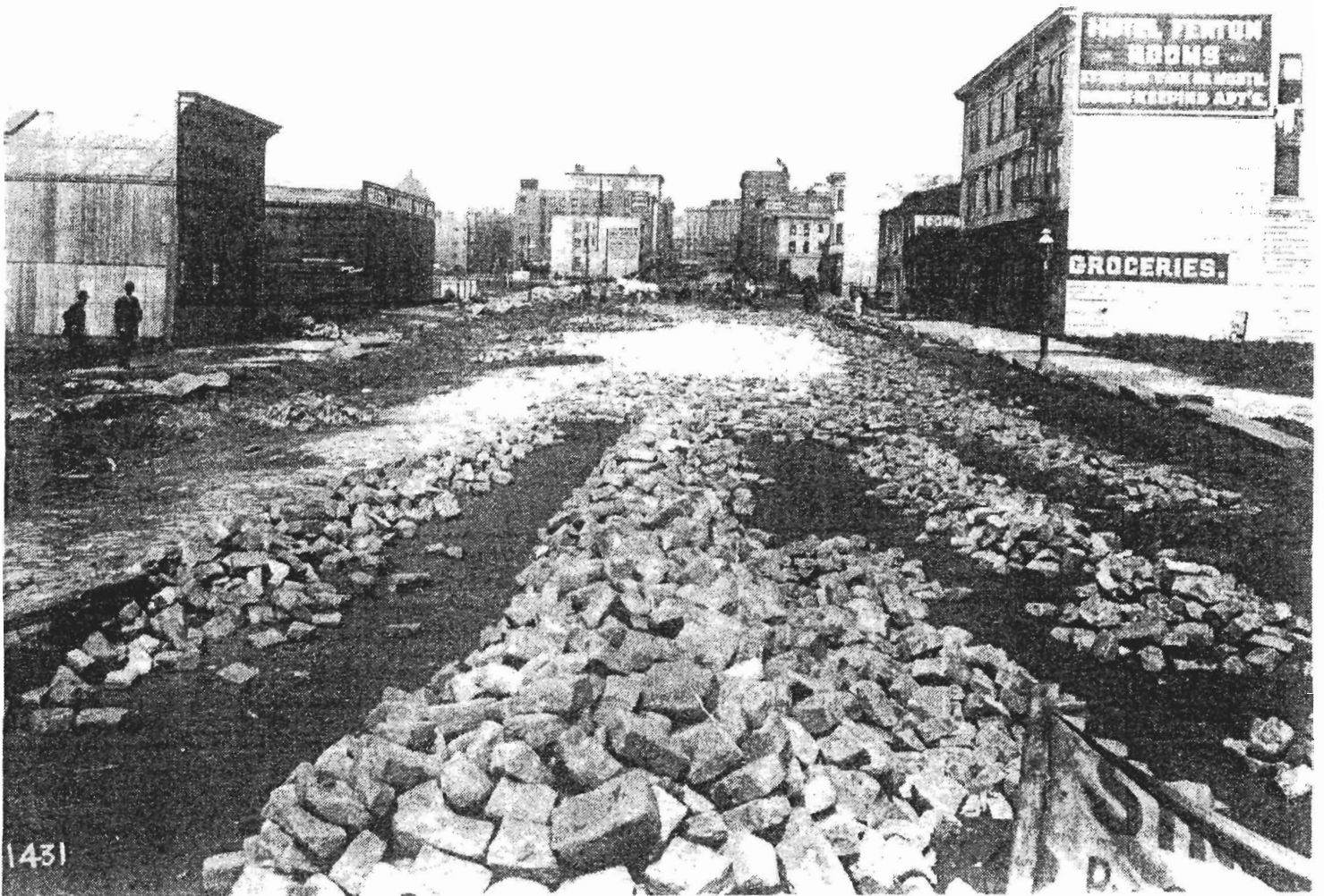
Hand-hewn Basalt Paving Blocks Ready to Be Laid on Seventh Street, North of Folsom, April 4, 1913: Considered "invincible street paving" by San Francisco's Superintendent of Public Streets in 1916—basalt blocks were comparatively expensive, $60 per thousand. At six cents a piece the stone mason kept 3.5 cents each, but after a strike he got 5 cents each. The rising cost of basalt paving, which had to include shipping and handling by rail and by water, made the far cheaper asphalt a bargain hard to resist especially as automobiles became less of a curiosity and drivers more demanding of smooth, quiet rides
