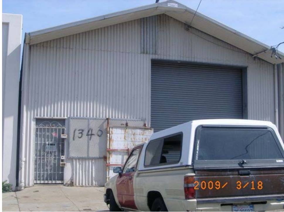
Donner Avenue near Ingalls Street: rusted and damaged siding.
