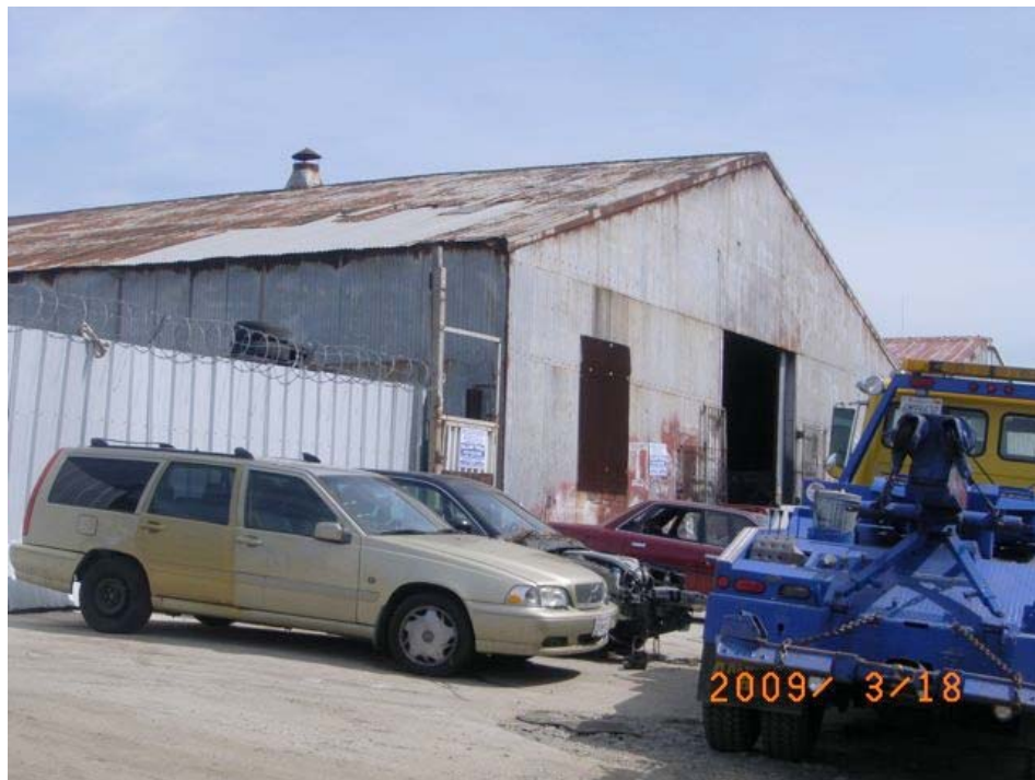
Underwood Avenue near Ingalls Street: deteriorated and rusted roofing and siding, razor wire security fence.
