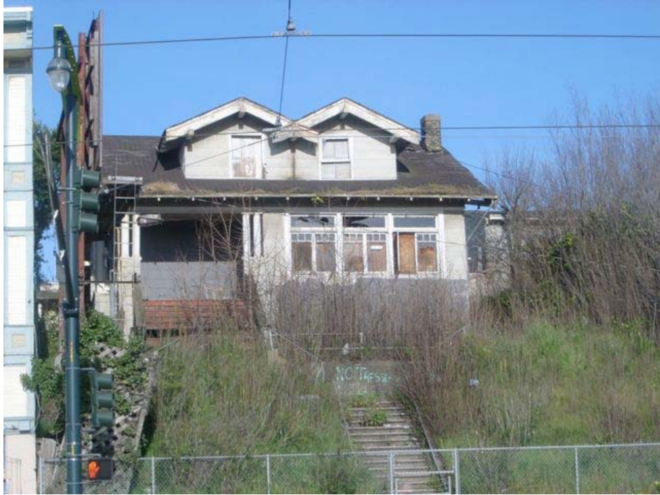
3 rd Street near Williams Avenue: extensive dilapidation, deteriorating roofing, broken and boarded windows, overgrown landscaping.
