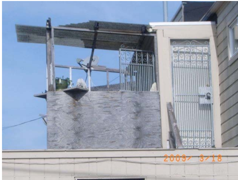
Jennings Street near Hollister Avenue: informal and substandard construction, deteriorated roofing, alignment problems.
