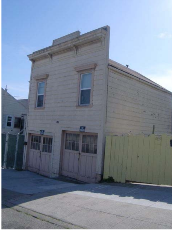
Phelps Street near Palou Avenue: deteriorated building, rotting garage door and peeling paint.
