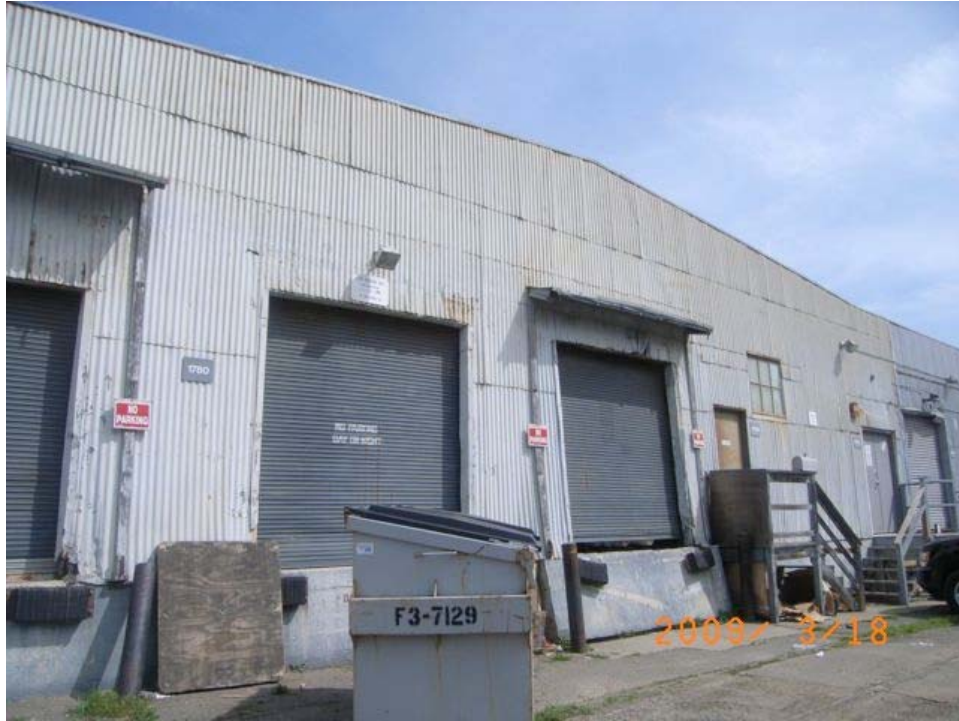
Armstrong Avenue and Mendell Street: industrial building with peeling paint, rusted siding, outdoor storage.
