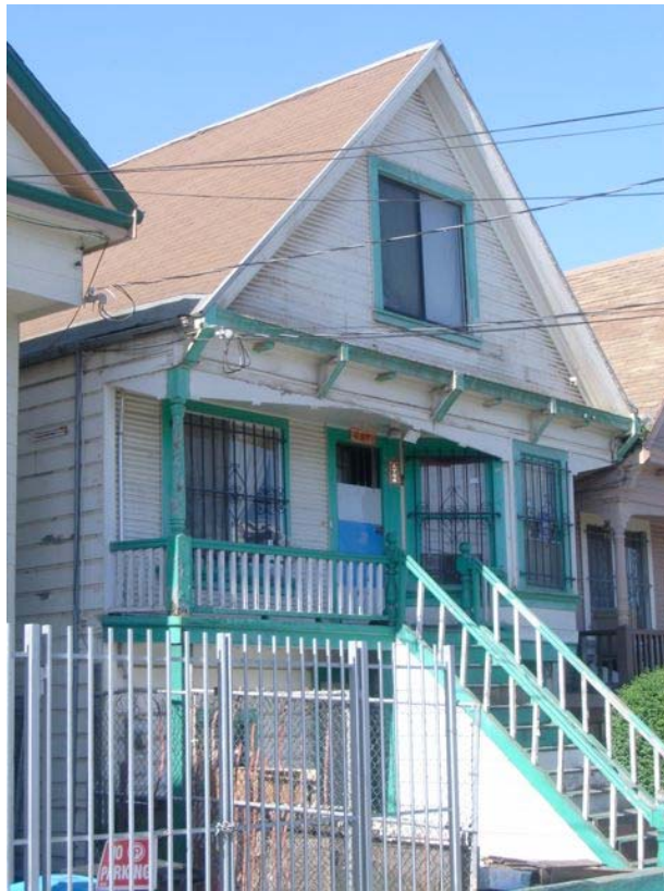
Kirkwood Avenue near Newhall Street: extensive deterioration, peeling paint, dry rot, informal and substandard construction, security bars.
