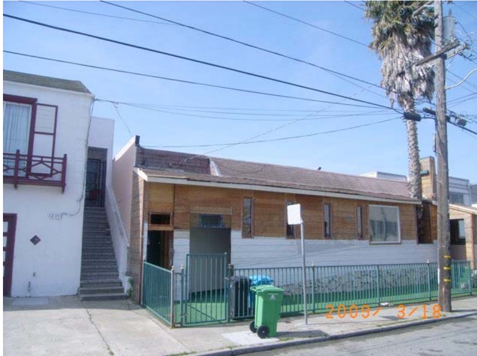
Egbert Avenue near Hawes Street: informal and substandard construction, sagging roof.
