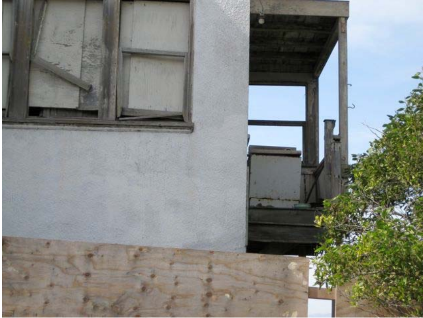
Newcomb Avenue near Lane Street: abandoned house, boarded windows, dry rot, outdoor storage, cracked wall, informal and substandard construction.
