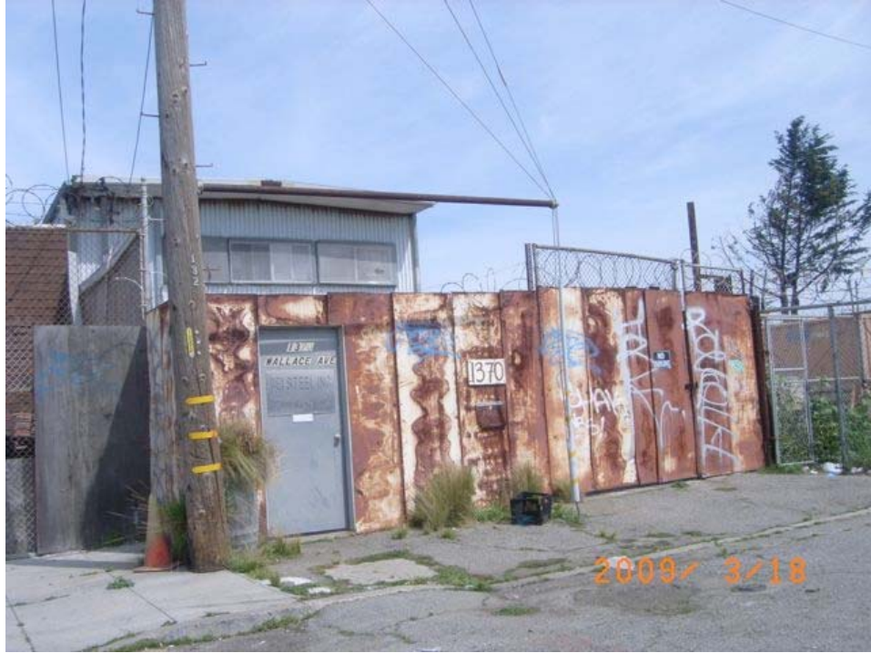
Wallace Avenue near Ingalls Street: informal and substandard construction, deteriorated sidewalk, extensive deferred maintenance, razor wire security fence, rusted gate.
