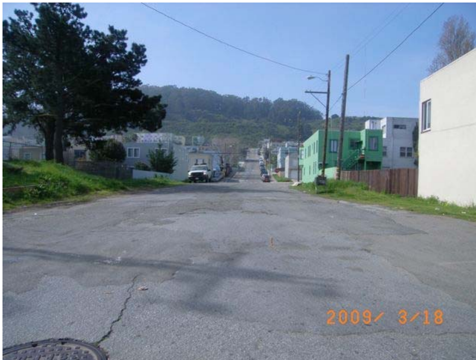
Hawes Street near Fitzgerald Avenue: deteriorated roadway, lack of sidewalks.
