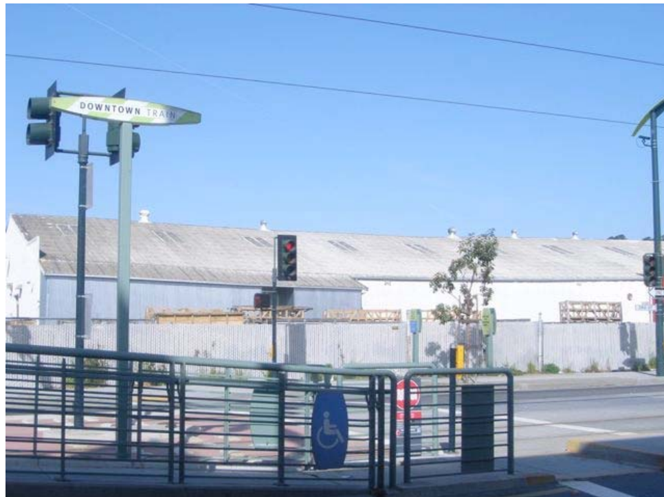
3 rd Avenue near Tulare Street: sagging roof.
