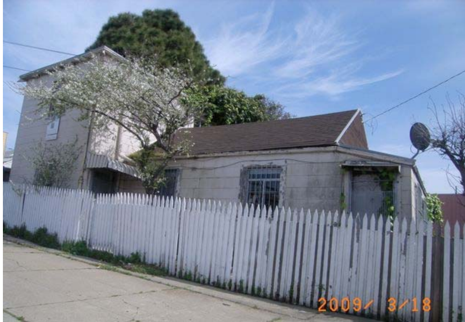
Keith Street near Underwood Avenue (different angle on property above): sagging roof, dry rot, deteriorated windows, deteriorated fence, external wiring, extensive deterioration.
