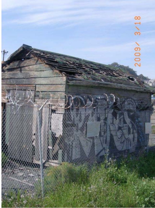
Indiana Street near Tulare Street: uninhabitable dilapidated building, collapsed roof, dry rot, peeling paint, graffiti.
