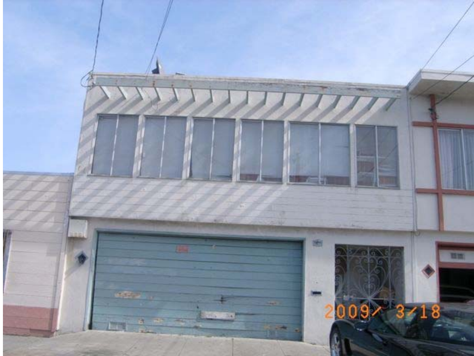
Fitzgerald Avenue near Ingalls Street: dilapidated garage door, extensive deterioration, older windows, peeling paint.
