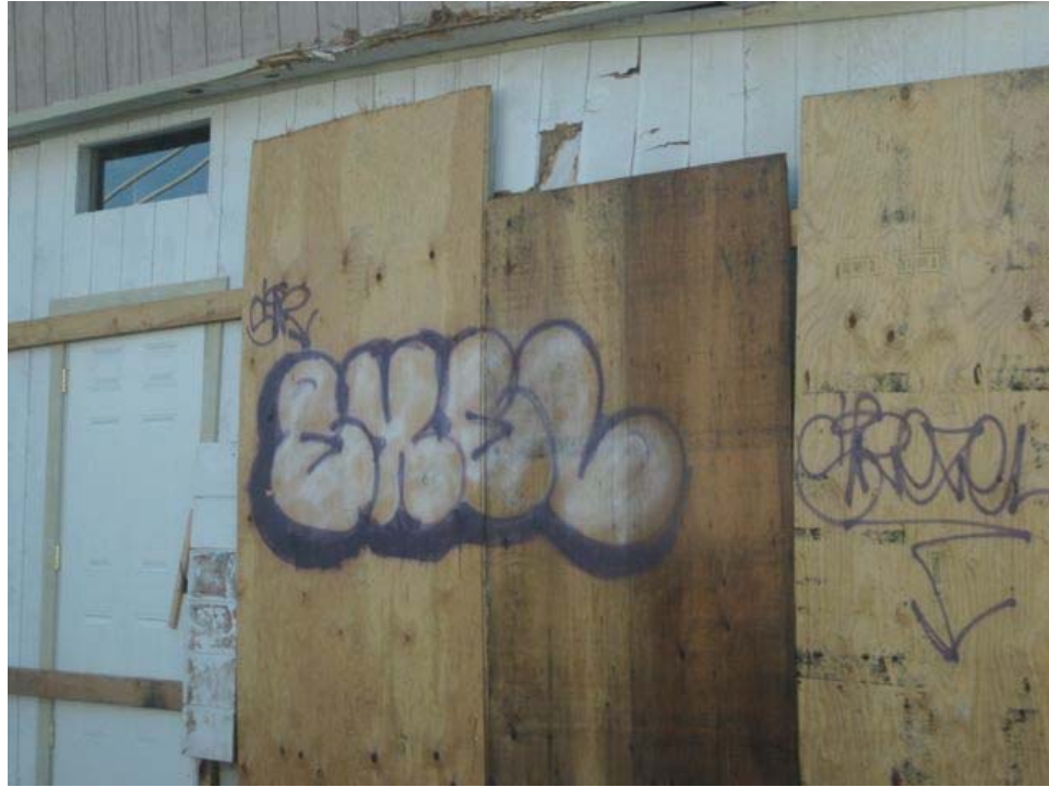
3 rd Street near Palou Avenue (close up of above): boarded windows, graffiti, deteriorating siding.
