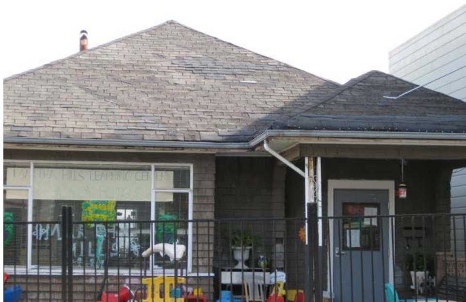
Jamestown Avenue near Jennings Street: deteriorating and water-damaged roofing.
