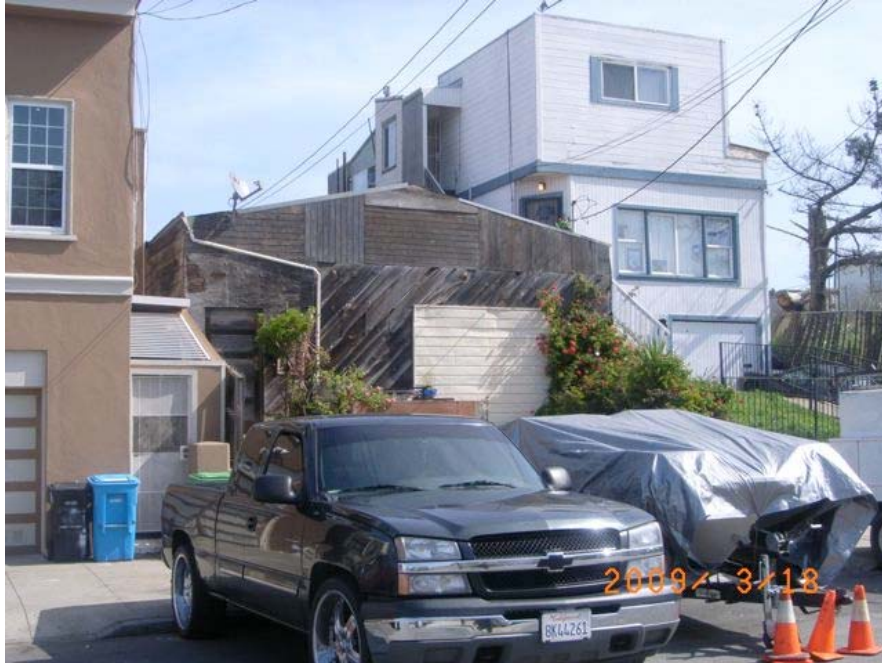
Egbert Avenue near Hawes Street: informal and substandard construction, water damage to wood siding.
