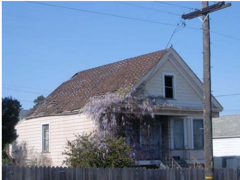
Oakdale Avenue near Quint Street: severely dilapidated building, sagging roof with large gaps, dry rot, broken windows.
