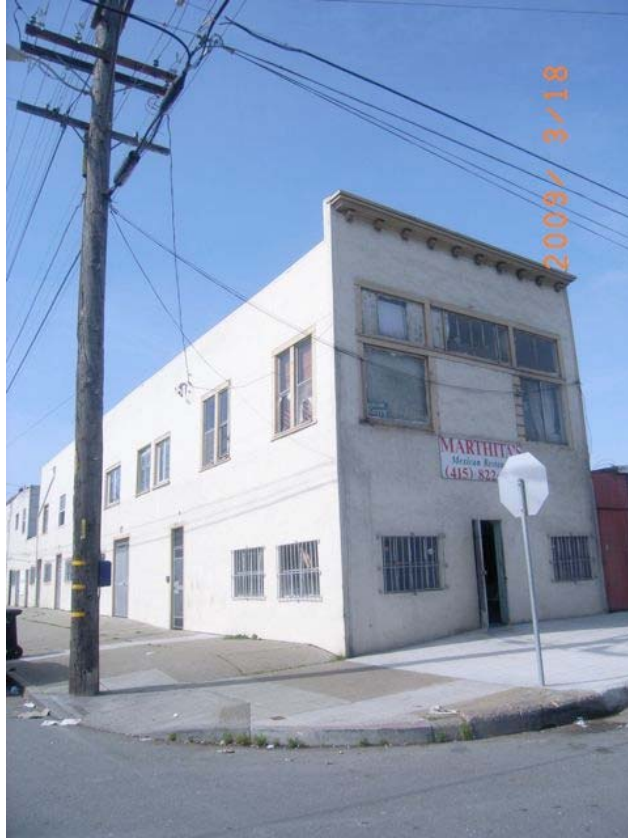
Egbert Avenue and Jennings Street: deteriorated, broken and boarded windows, informal external wiring, peeling paint.
