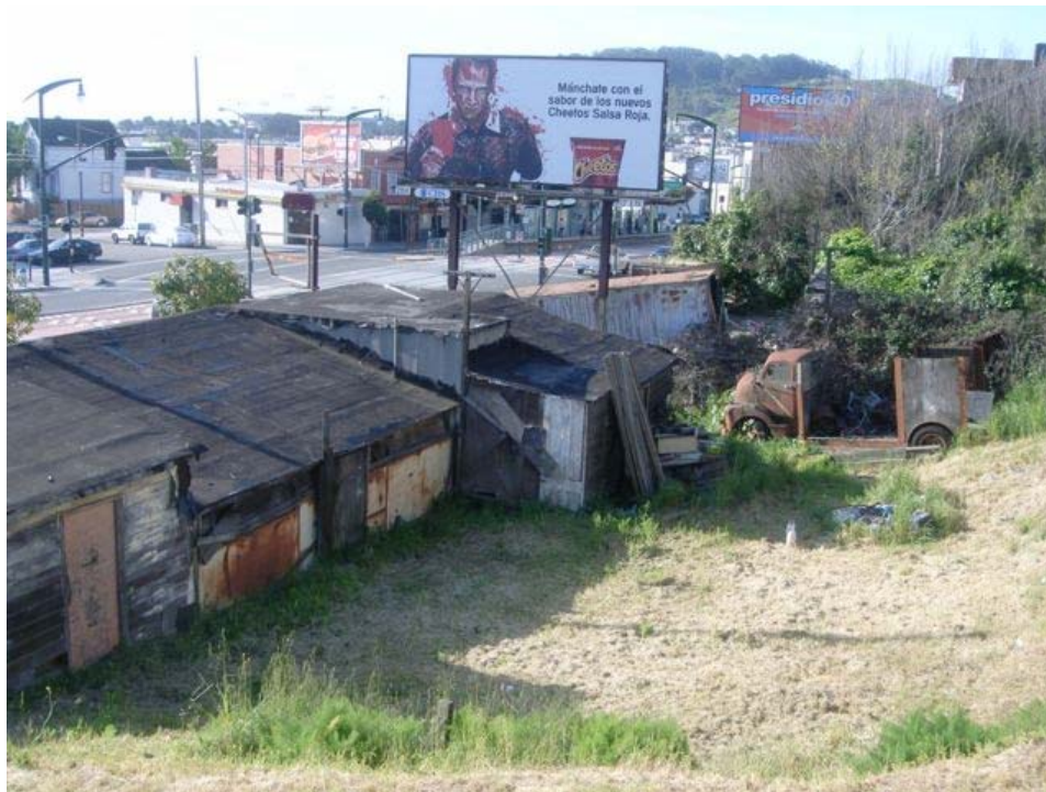
3 rd Street at Thornton Avenue, rear: extensive dilapidation, deteriorating roof and walls, substandard and informal construction, outdoor trash dumping.
