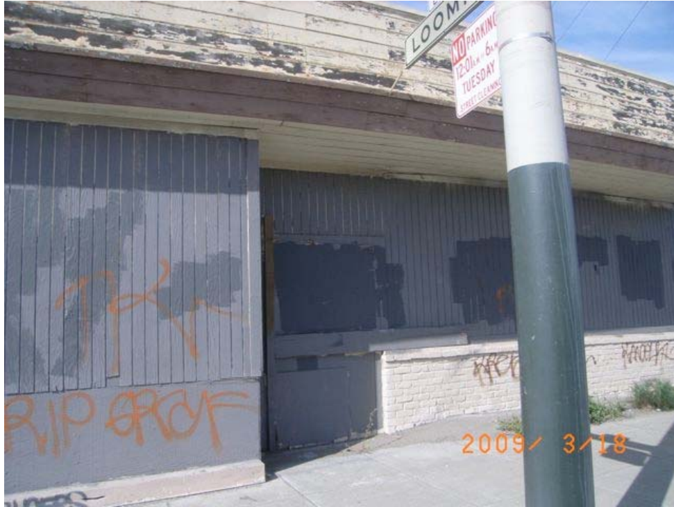
Industrial Street near Loomis Street (close up of above): vacant and dilapidated building, peeling paint, dry rot, graffiti.
