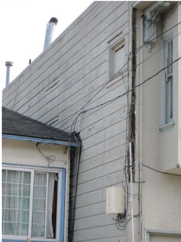
Hollister Avenue near Hawes Street: extensive deferred maintenance, evidence of dry rot, deteriorated siding, external wiring.
