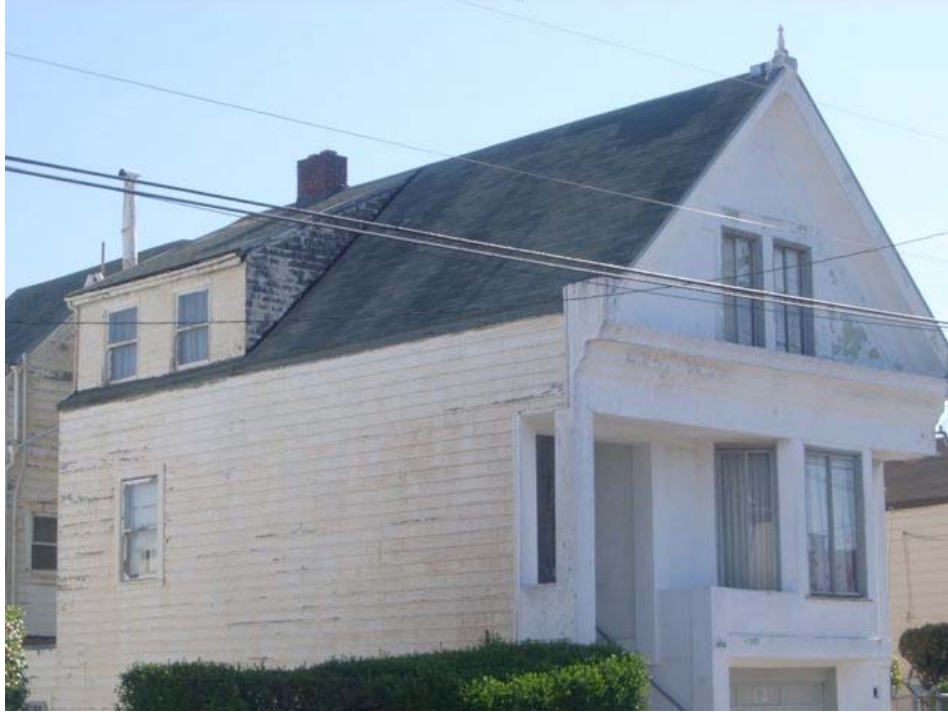
Kirkwood Avenue near Newhall Street: peeling paint, dilapidated siding, extensive deterioration.
