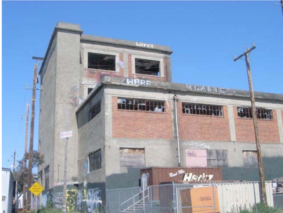
Davidson Avenue near Rankin Street: vacant and severely dilapidated industrial building, broken and boarded windows, graffiti, unreinforced masonry.
