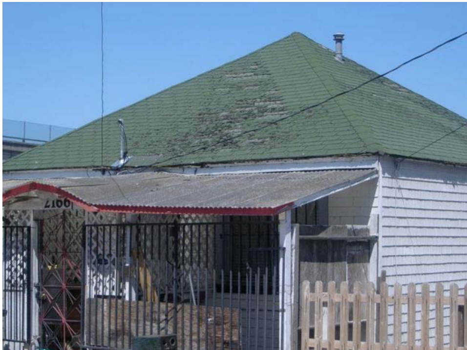
Revere Avenue near I-280: dilapidated building, dry rot deteriorating roofing, informal and substandard construction.
