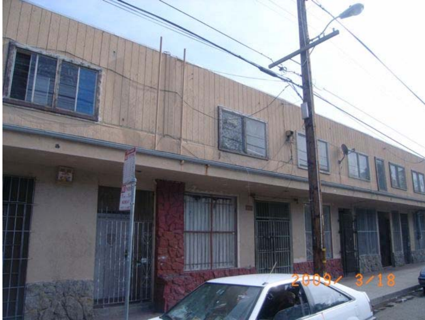
Gilman Avenue near Griffith Street: extensive siding deterioration, peeling paint, water damage, external wiring, security doors, deteriorated older windows.
