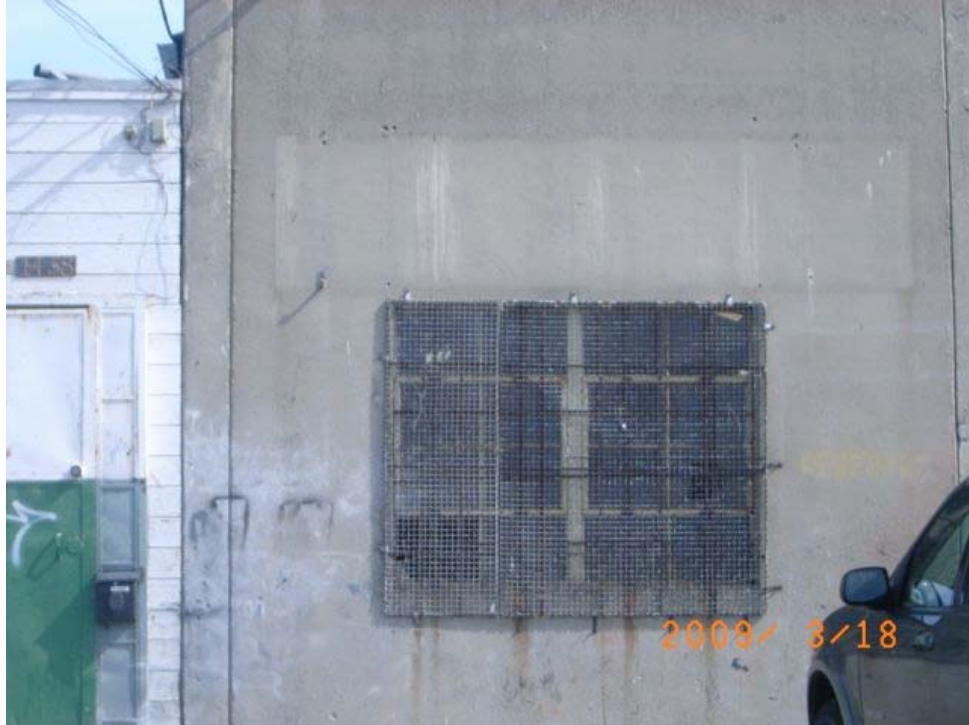
Egbert Avenue near Jennings Street: security grate, graffiti, water damage.
