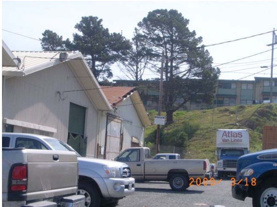
Donner Avenue near Hawes Street: deteriorated roof and siding, rusted door.
