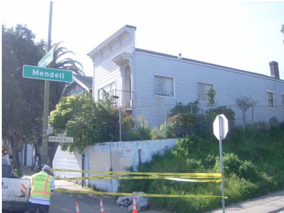
Hudson Avenue at Mendell Street: cracked and leaning retaining wall, extensive deterioration, water damage, boarded window.
