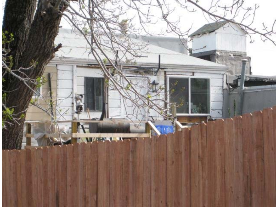
Hollister Avenue near Hawes Street: peeling paint, dry rot, cracked siding, informal and substandard construction.
