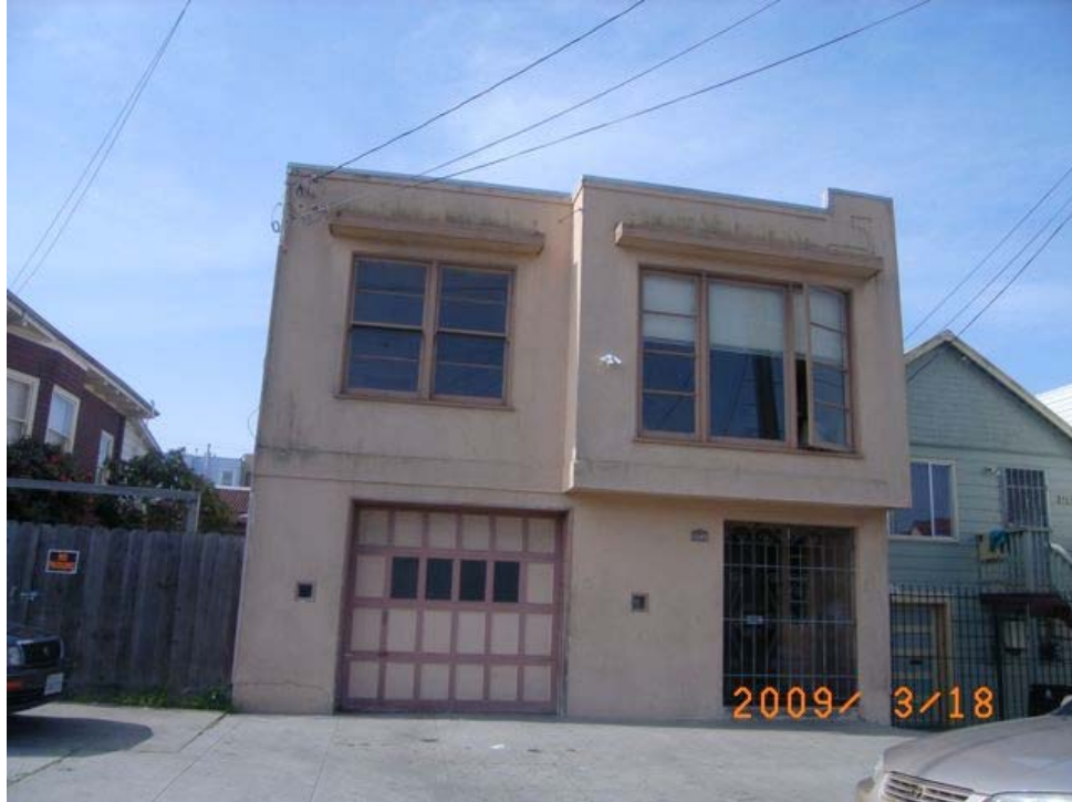
Hollister Avenue near Jennings Street: Cracked wall, water damage, older windows.
