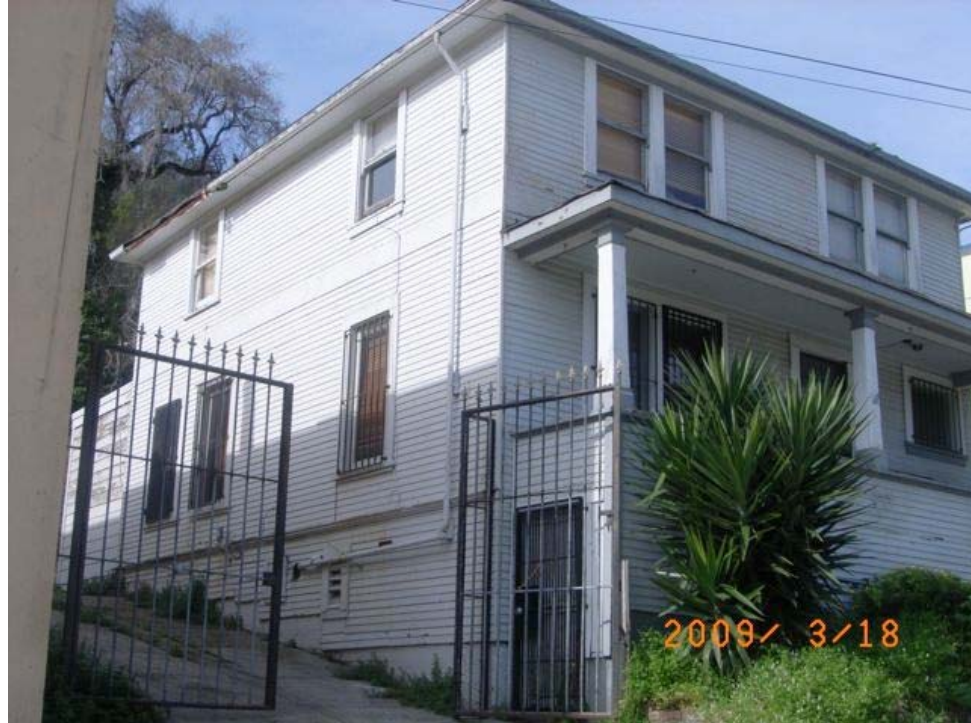
Ignacio Avenue near Ingerson Avenue: deteriorated siding, damaged gutters, peeling paint, security grates.
