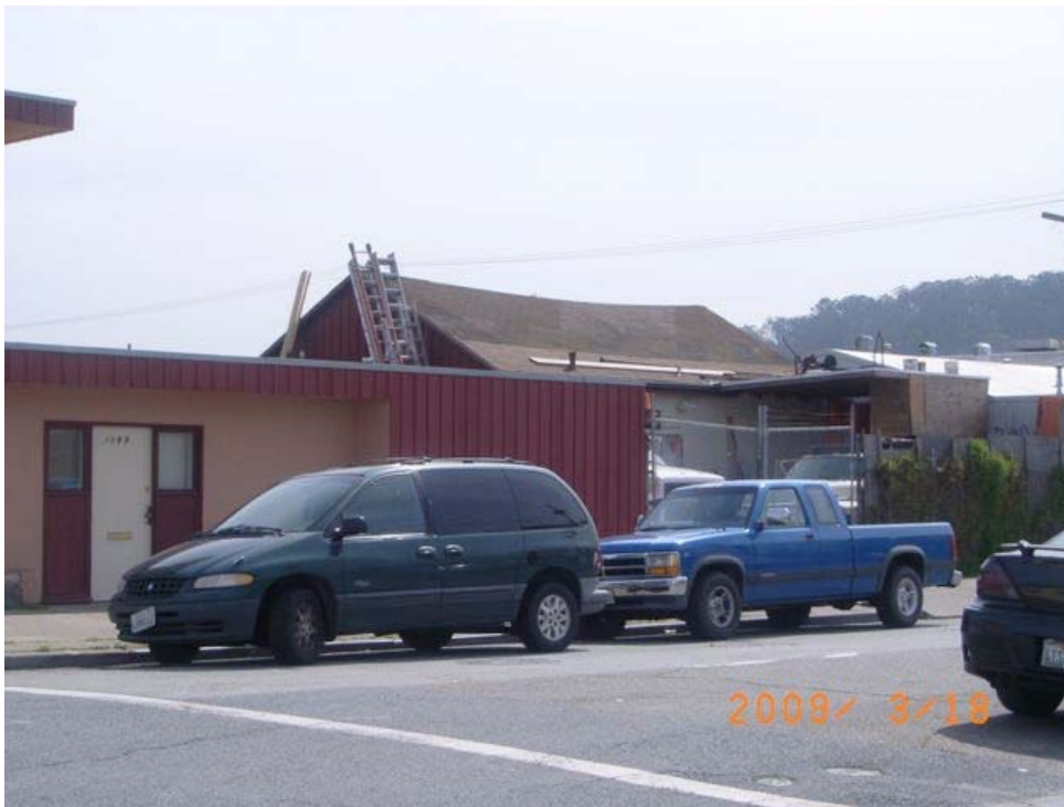
Van Dyke Avenue near Keith Street: sagging roof, informal and substandard construction.
