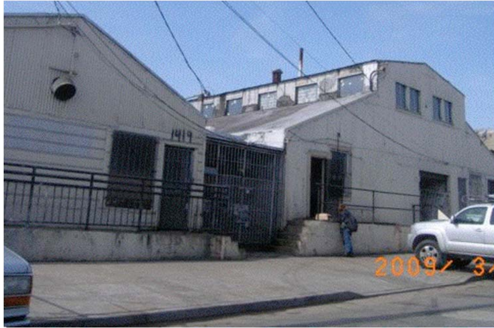
Egbert Avenue near Jennings Street: deteriorated roofing and siding, peeling paint, water damage.
