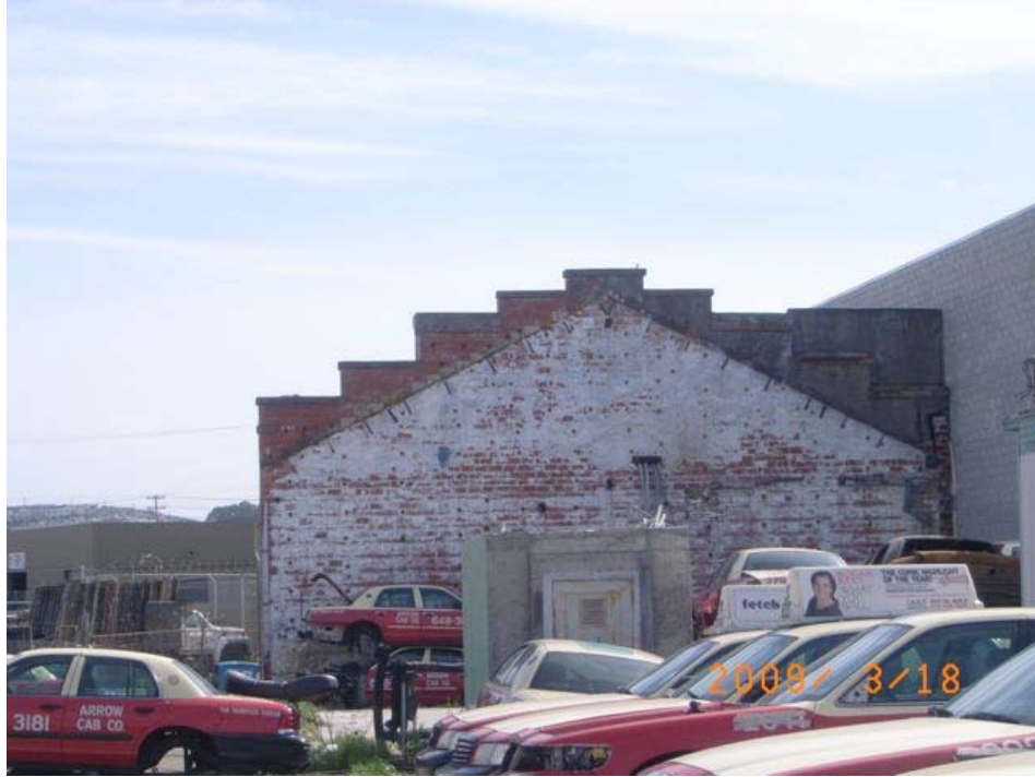
Marin Street near Jerrold Avenue: outdoor storage, unreinforced masonry construction, extensive deterioration.
