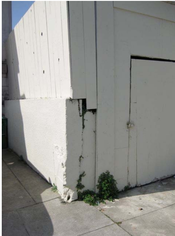
Egbert Avenue near Hawes Street: cracking foundation wall, rotting wood, alignment problems.
