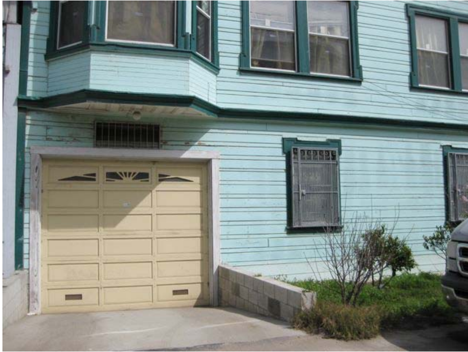
Armstrong Avenue near 3 rd Street: informal external wiring, peeling paint.
