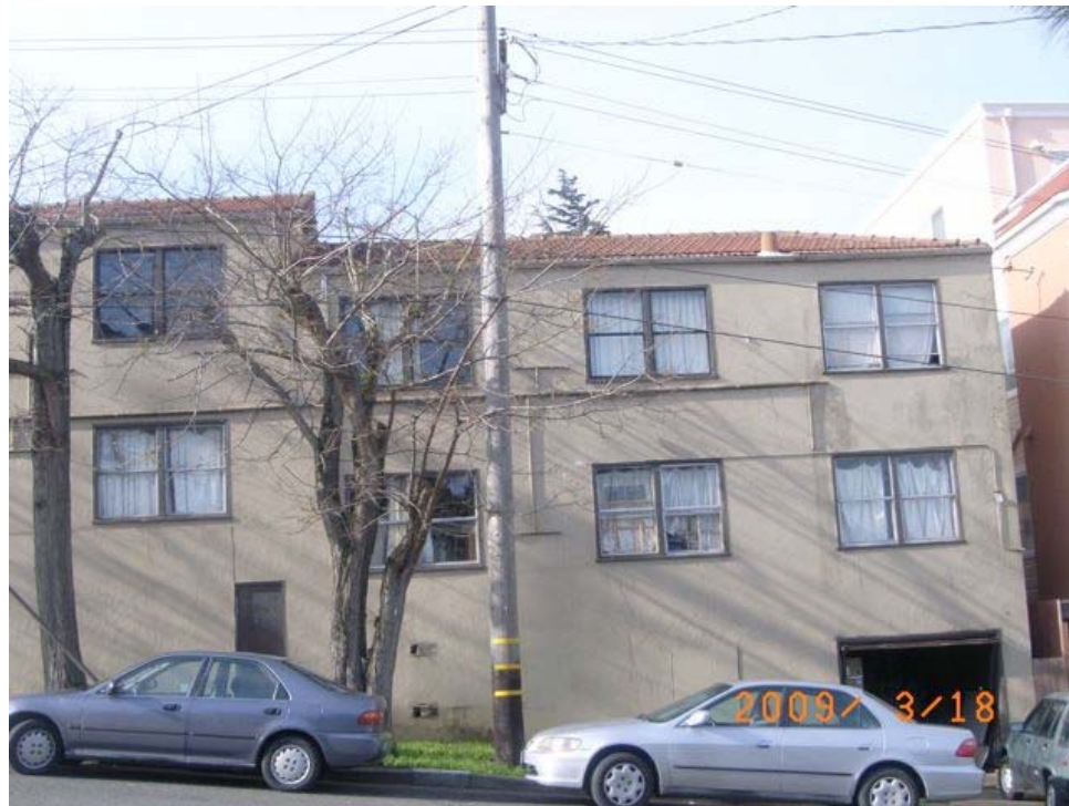
LeConte Avenue near 3 rd Street: deferred maintenance and broken windows.
