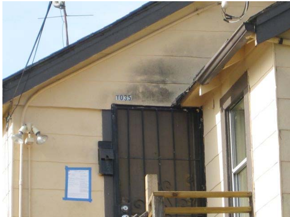
Ingerson Avenue near Ingalls Street (close up of above): smoke damage, broken/missing eave.
