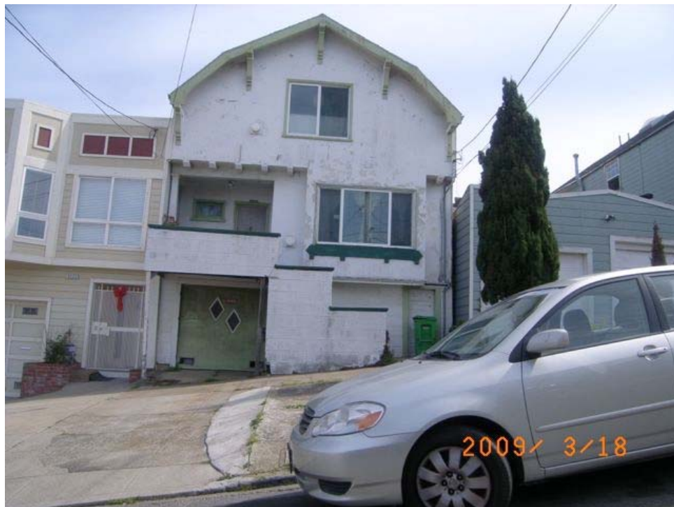
Jennings Street near Ingerson Avenue: extensive deterioration, peeling paint, water damage.
