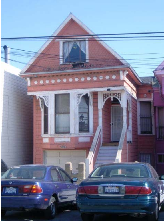
Newcomb Avenue near Newhall Street: cracked wall, peeling paint, evidence of dry rot.
