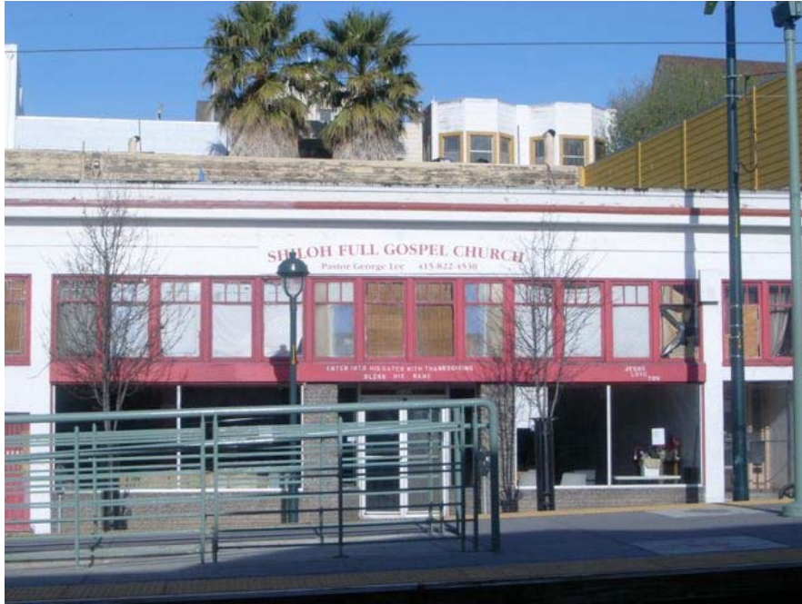
3 rd Street near Shafter Avenue: deferred maintenance, boarded window, cracked wall.
