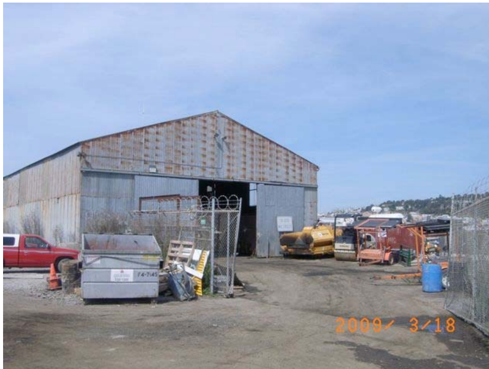
Armstrong Avenue at Griffith Street: rusted and deteriorated siding, outdoor storage, lack of sidewalks.
