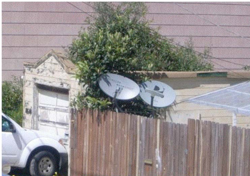
Revere Avenue near I-280: peeling paint, sagging roof, extensive deferred maintenance.
