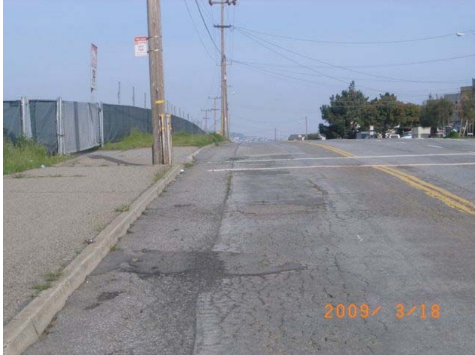
Jamestown Avenue near Ignacio Avenue: deteriorated pavement, cracked sidewalk, overgrown grass on sidewalk.
