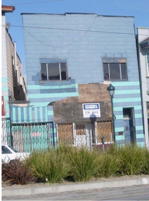
3 rd Street near Oakdale Avenue: informal and substandard construction, extensive dilapidation, missing siding, boarded windows and door, alignment problems, water damage.
