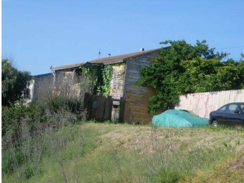
3 rd Street at Thornton Avenue: extensive deferred maintenance, peeling paint, graffiti, deteriorating roof and eaves,
