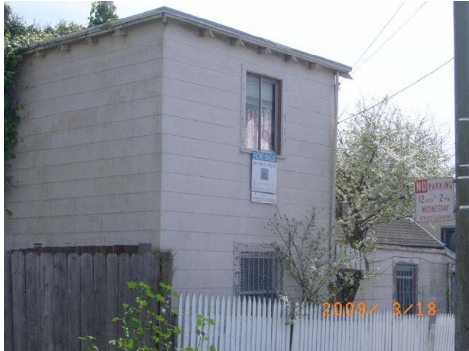
Keith Street near Underwood Avenue: peeling paint, sagging roof, dry rot, extensive deterioration of smaller building, missing eaves.
