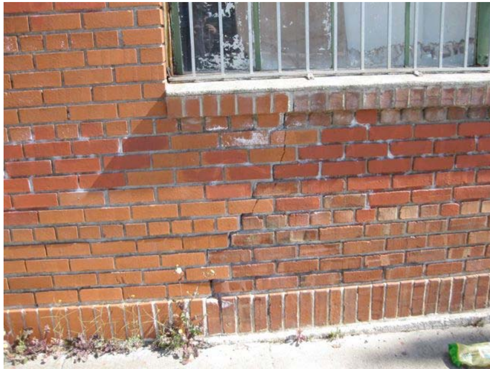
Evans Avenue near Quint Street: cracked brick wall.
