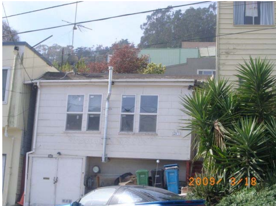
Ignacio Avenue near Ingerson Avenue: informal and substandard construction, sagging roof, alignment problems, faded paint.
