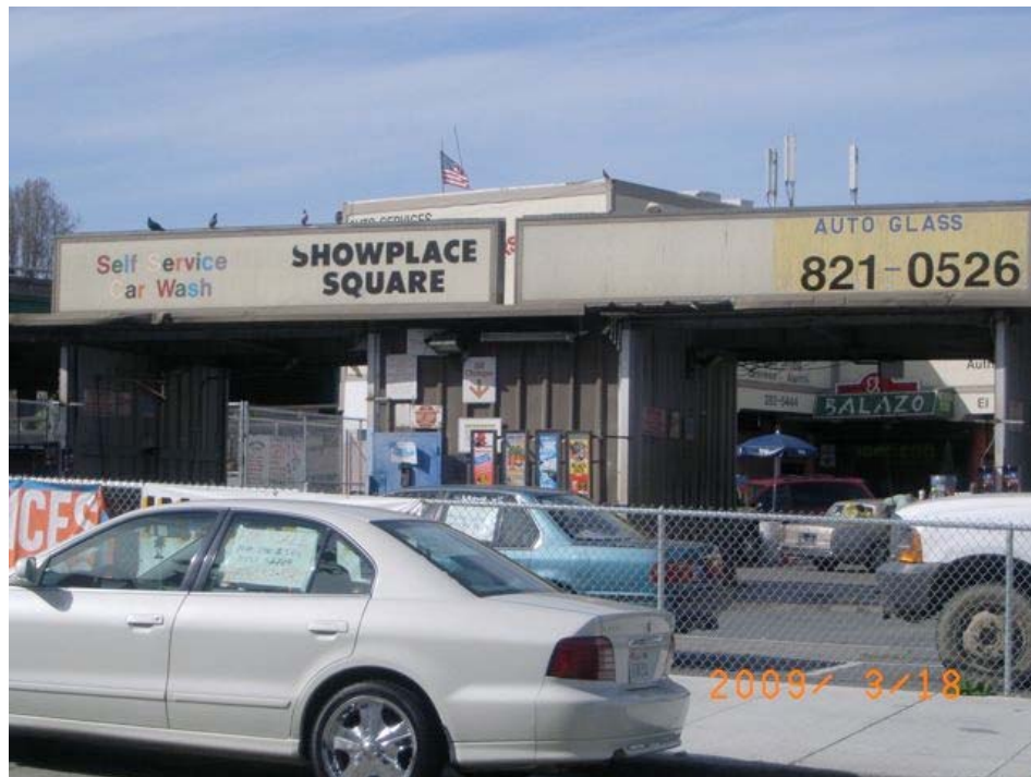
Marin Street near Bayshore Boulevard: deteriorated roofing and signage.
