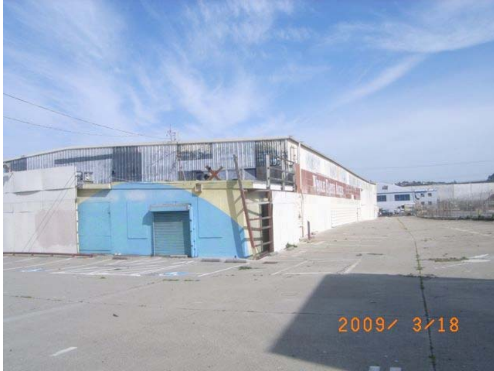
Bayshore Boulevard near Cortland Avenue: vacant building, informal and substandard construction, extensive deterioration, peeling paint.
