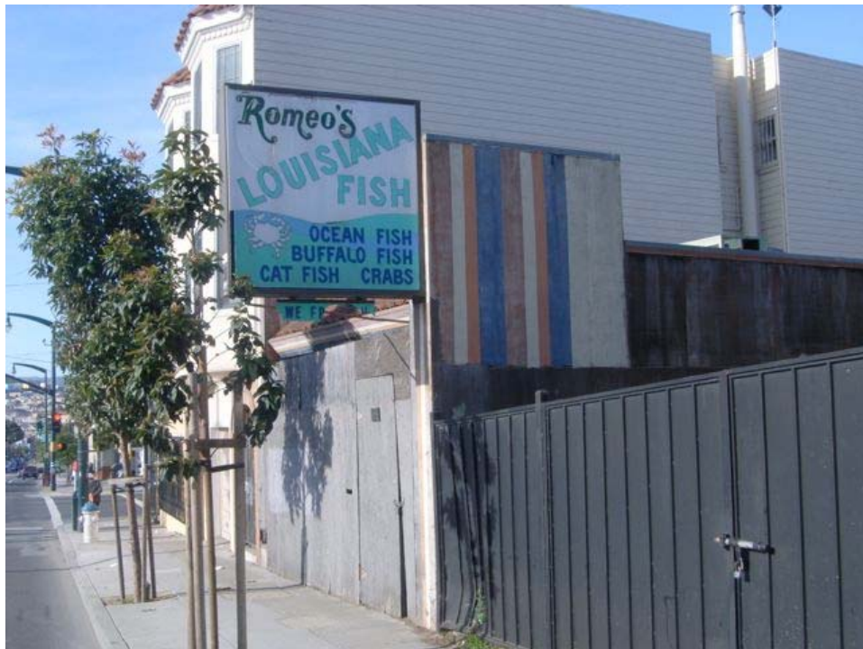
3 rd Street near Williams Avenue: abandoned business space, boarded storefront, extensive deterioration, informal and substandard construction.
