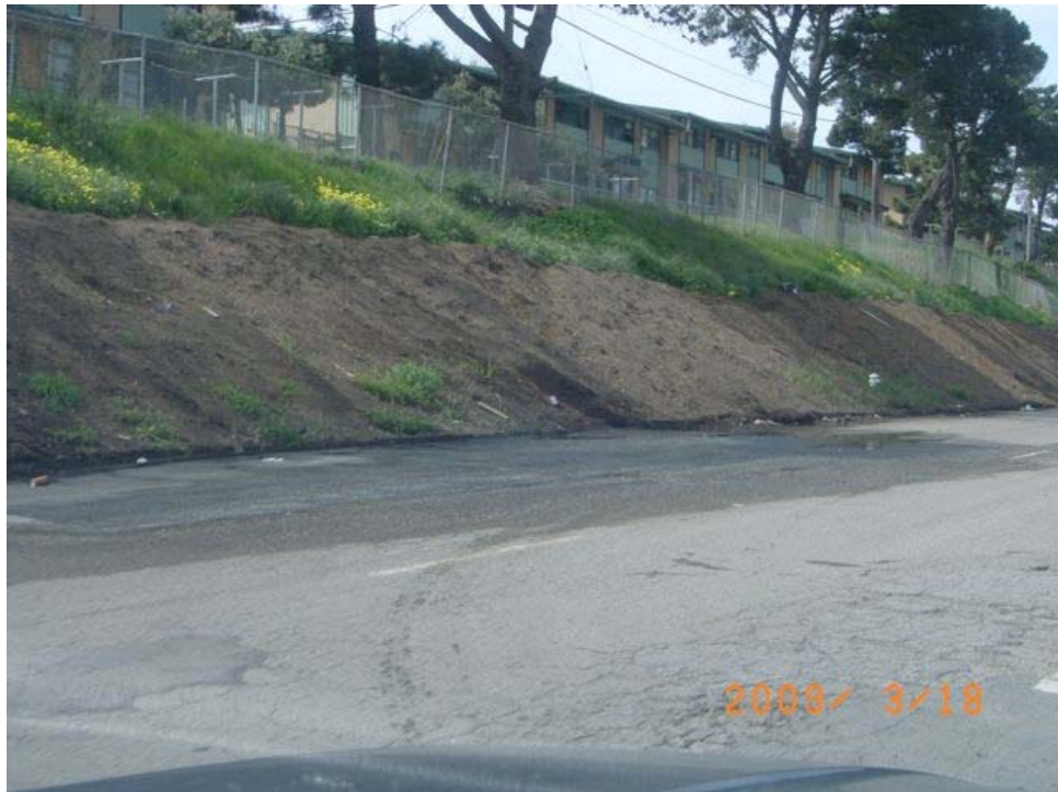
Carroll Avenue near Arelious Walker Drive: eroding hillside with inadequate grading; lack of sidewalk, curb or gutters; standing water; and trash accumulation.
