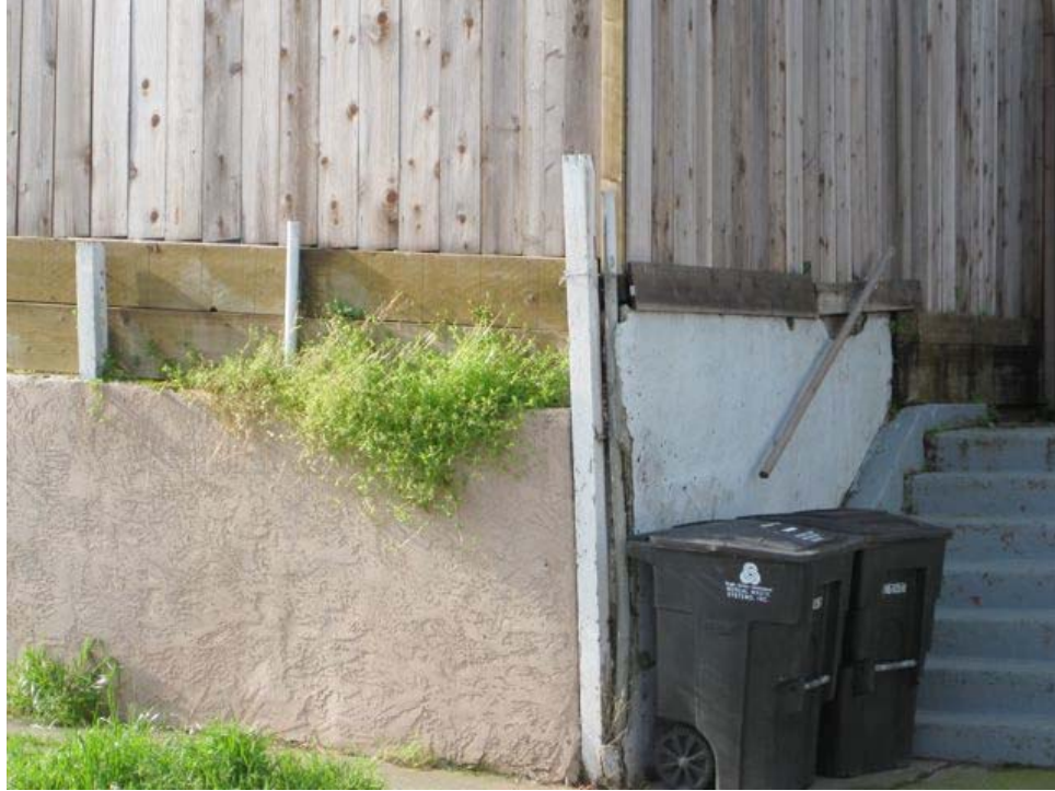
Key Avenue near 3 rd Street (close up of above): cracked retaining wall, overgrown landscaping, informal and substandard construction.
