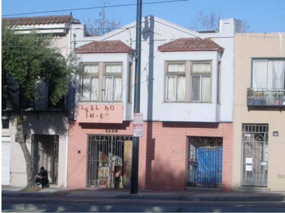
3 rd Street near Yosemite Avenue: deferred maintenance, deteriorated sign, outdoor storage.
