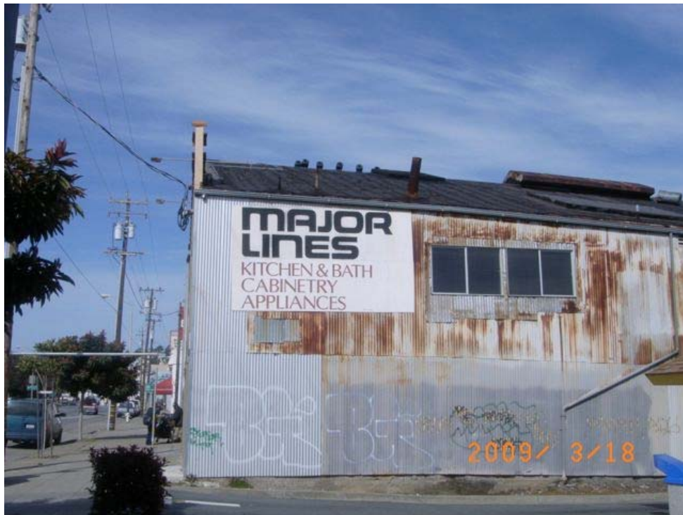
Bayshore Boulevard near Costa Street: eroded foundation, rusted and deteriorated siding, damaged roof, extensive deterioration, informal and substandard construction.
