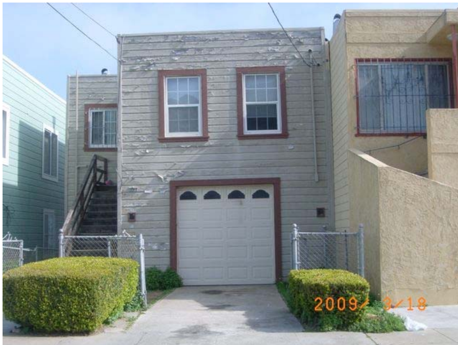
Hollister Avenue near Hawes Street: severely weathered siding.
