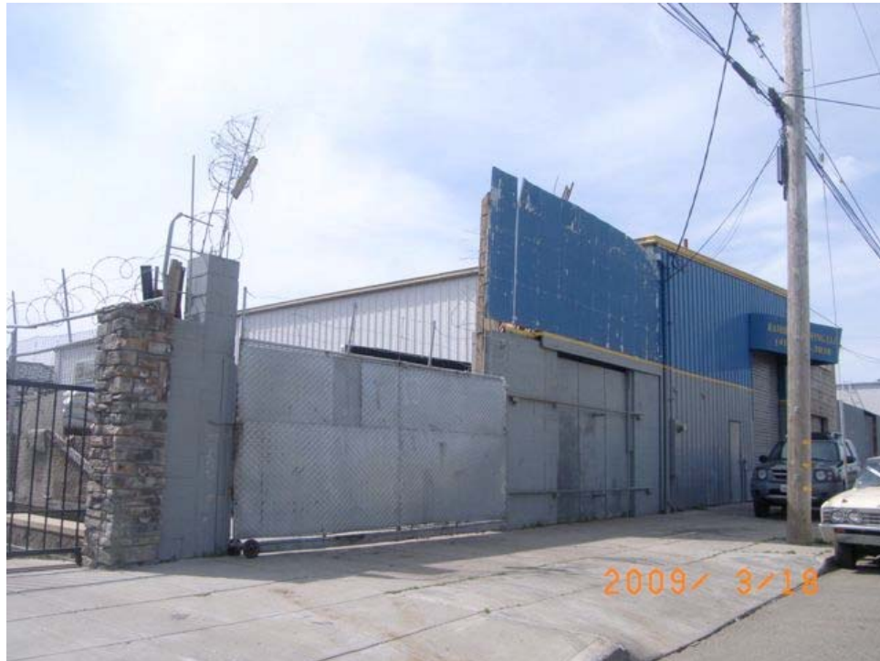
Thomas Avenue near Ingalls Street: severely deteriorated façade, informal and substandard construction, peeling paint, razor wire security fence.
