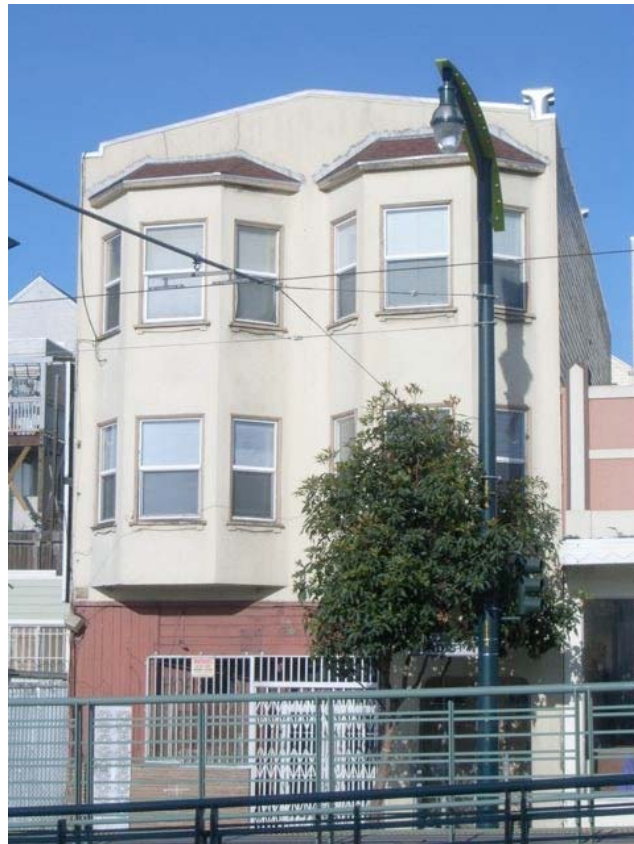
3 rd Street near Shafter Avenue: deteriorated siding, cracked wall, external wiring, peeling paint.
