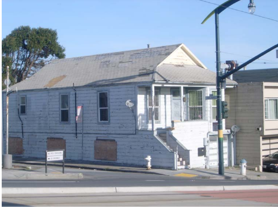
3 rd Street at Salinas Avenue: extensive dilapidation, peeling paint, boarded windows, deteriorating roofing and eaves.
