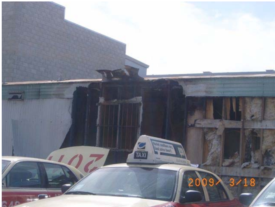
Marin Street near Jerrold Avenue: fire damage, extensive dilapidation, broken/missing windows.
