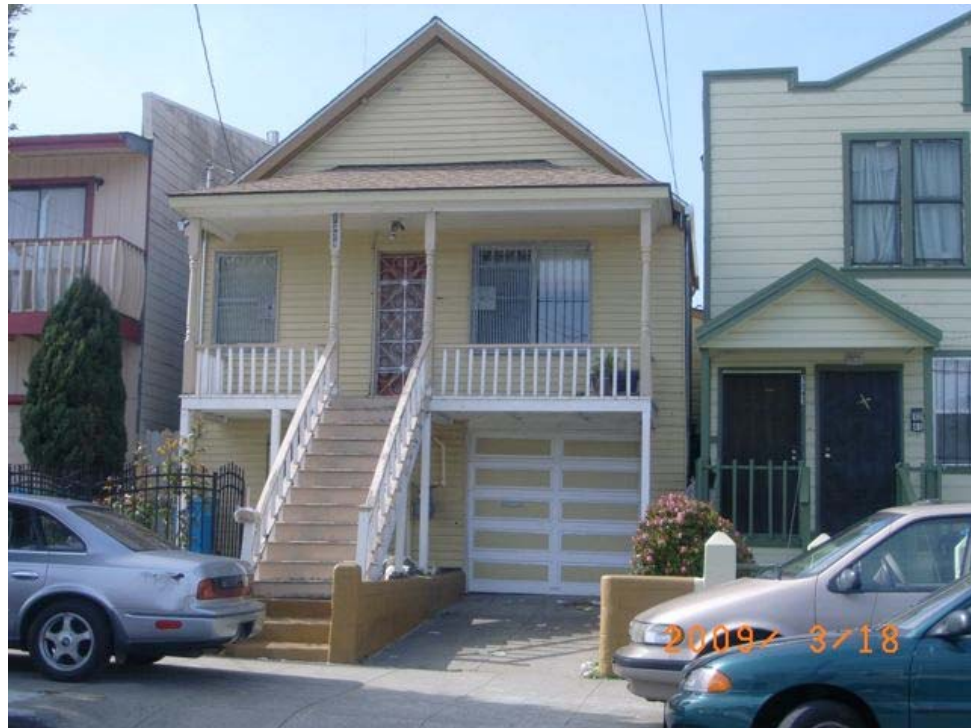
Gilman Avenue near Ingalls Street: deteriorated staircase, peeling paint, security grates.
