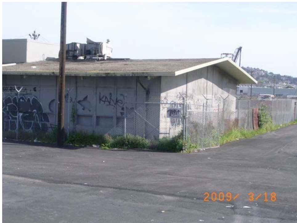
Cesar Chavez Street near I-280: graffiti, broken and boarded windows, barbed wire security fencing, extensive dilapidation.
