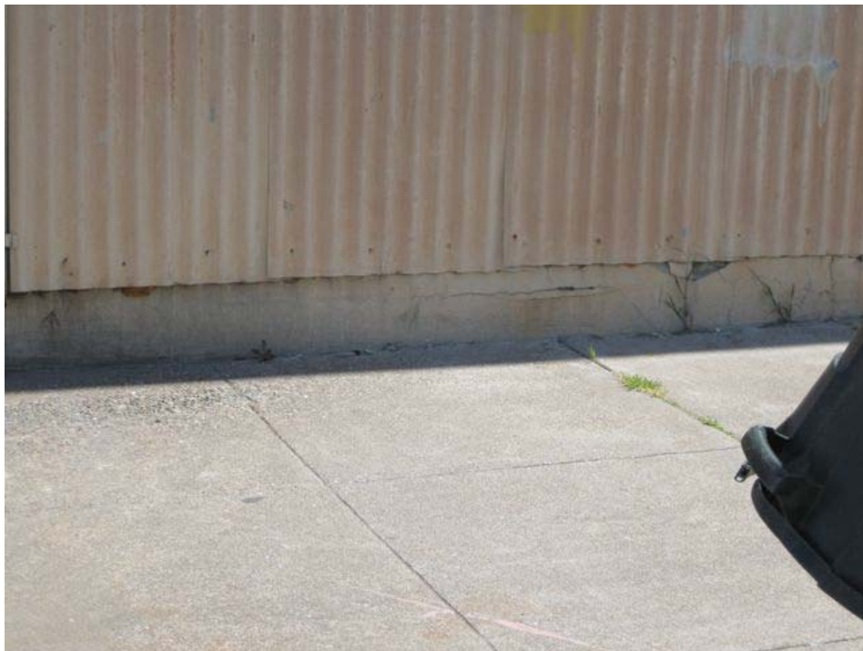
Kirkwood Avenue near Rankin Street: cracked foundation.
