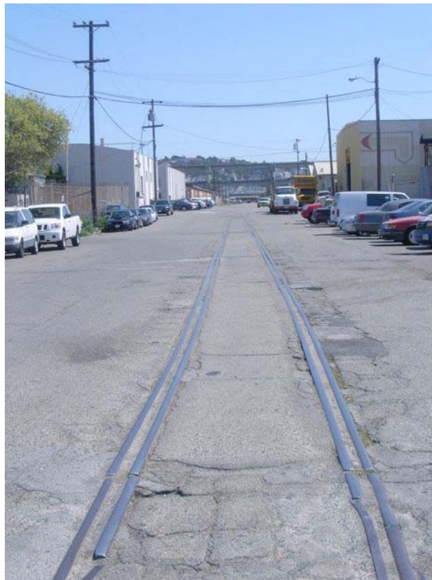
McKinnon Avenue near Barneveld Avenue: cracked pavement, abandoned rail line, lack of sidewalks.
