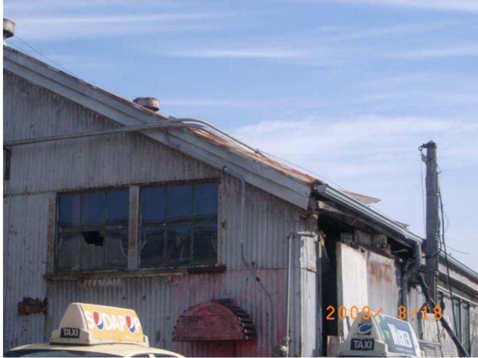
Marin Street near Jerrold Avenue: extensive dilapidation, informal and substandard construction, broken windows, graffiti, deteriorated roofing.
