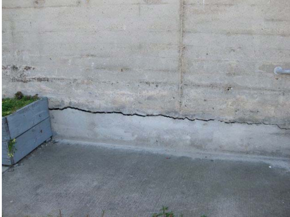
Toland Street near Galvez Avenue: cracked foundation.
