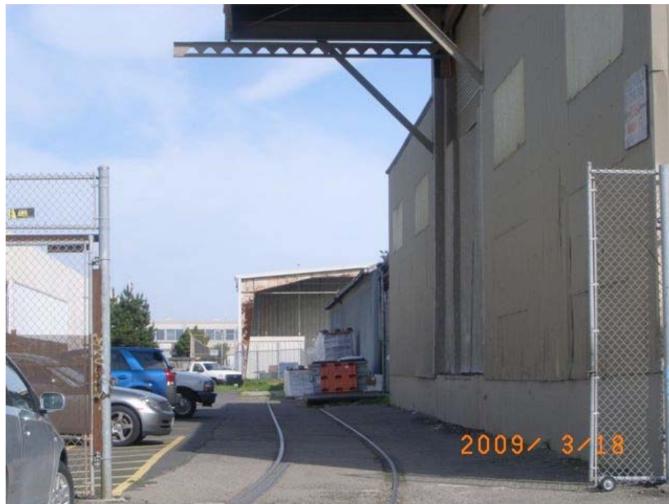
Michigan Street near Marin Street: abandoned railroad tracks, deteriorated siding.
