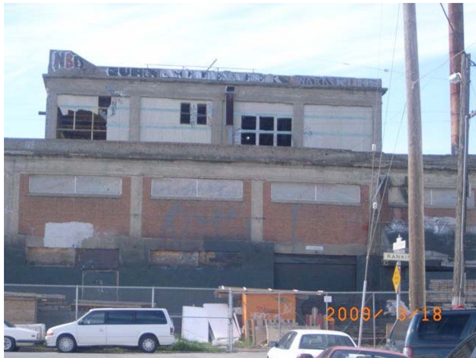
Custer Avenue near Rankin Street: abandoned building, cracked wall, fire damage, broken windows, extensive dilapidation, outdoor storage, graffiti.
