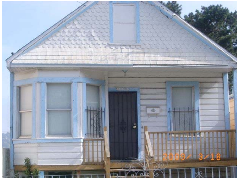
Hollister Avenue near Ingalls Street: deteriorated siding, security door, peeling paint, missing cripple wall.
