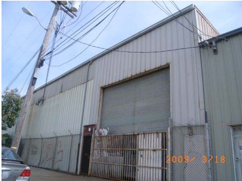
Ingalls Street near Bancroft Avenue: rusted and deteriorated siding, graffiti, security and barbed wire.
