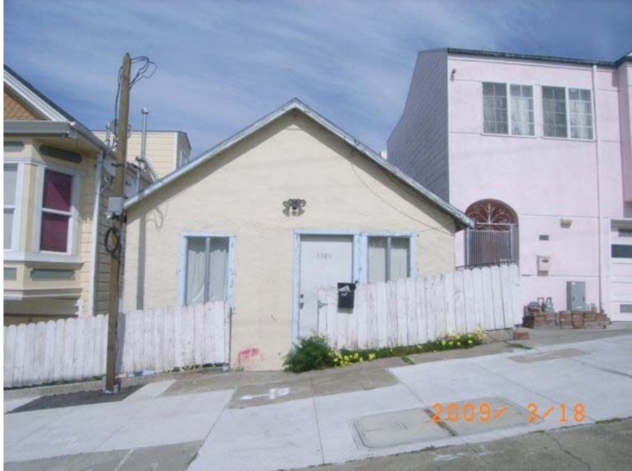
Newcomb Avenue near Lane Street: peeling paint, cracked foundation, deteriorated eaves.
