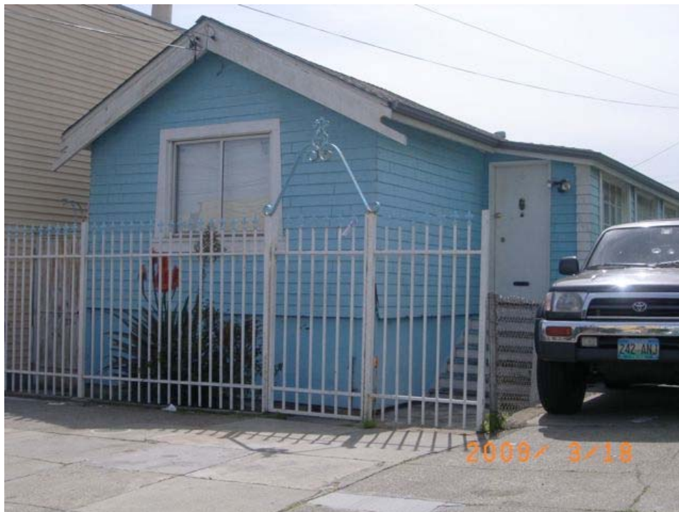
Shafter Avenue near Hawes Street: peeling paint, deteriorating siding.
