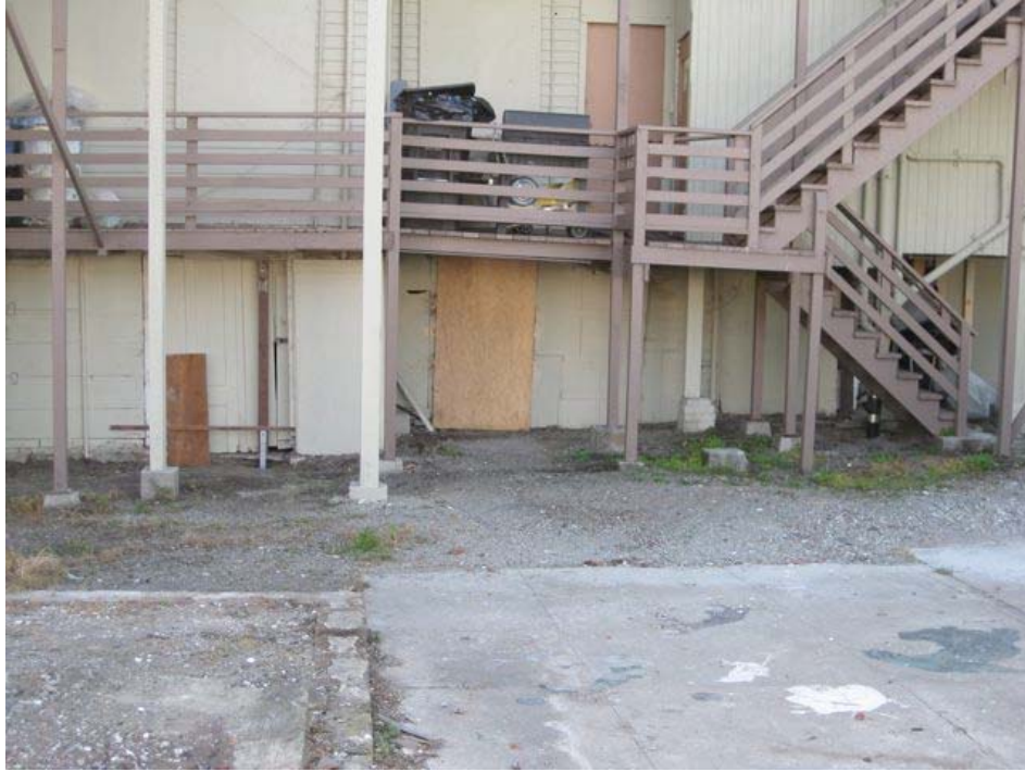
Newhall Street near LaSalle Avenue: informal and substandard construction, alignment problems, boarded doors.
