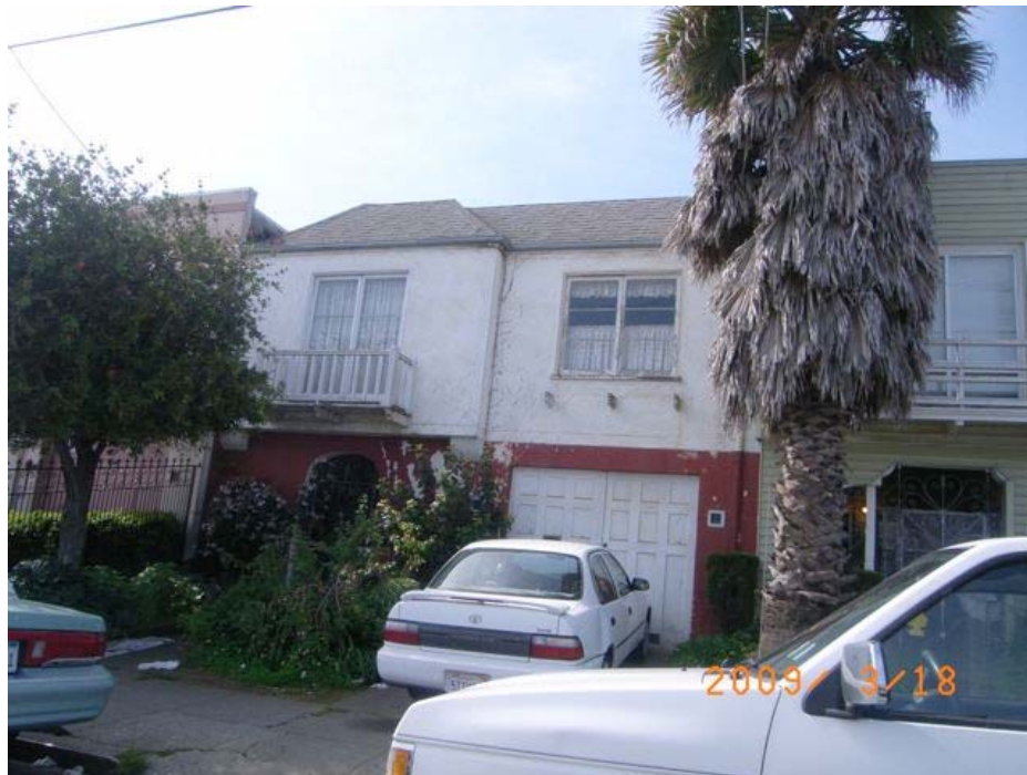
Fitzgerald Avenue near Jennings Street: deferred maintenance, evidence of dry rot, peeling paint.
