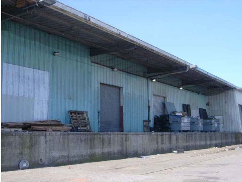
Innes Avenue near Rankin Street: deterioration, outdoor trash accumulation.
