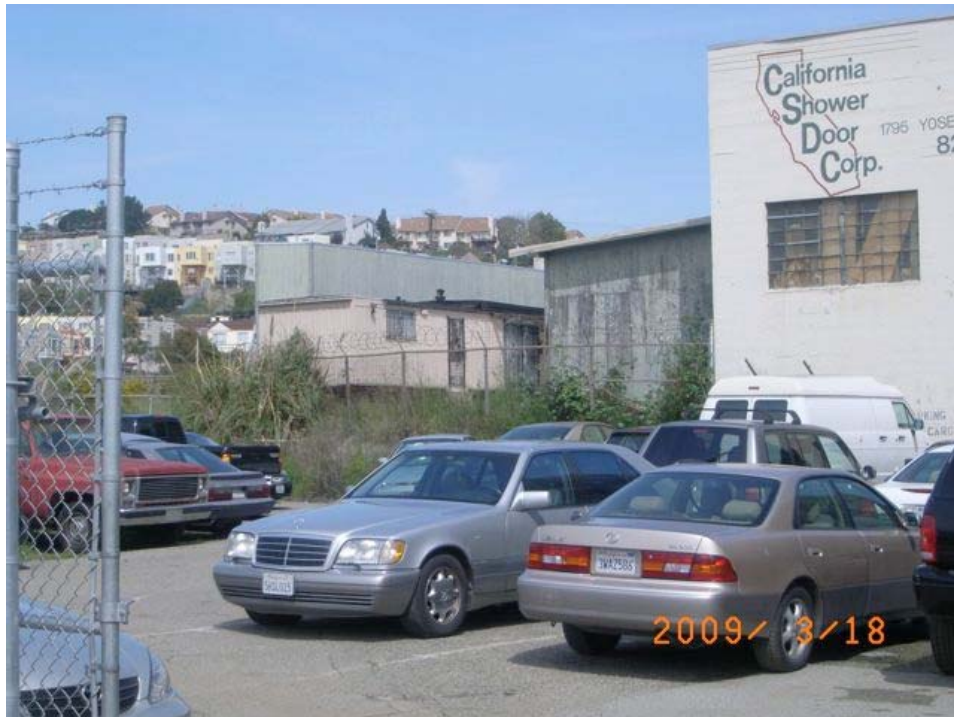
Armstrong Avenue near Mendell Street: peeling paint and deteriorated doors and windows. Shed shows signs of water damage and rotting wood.
