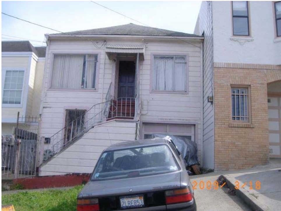
Jennings Street near Ingerson Avenue: peeling paint, deteriorated roofing, older windows.
