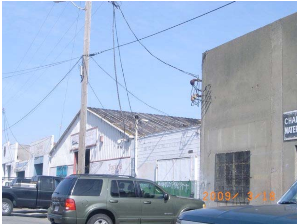
Egbert Avenue near Jennings Street: deteriorated metal roof, damaged siding, security grate, graffiti.
