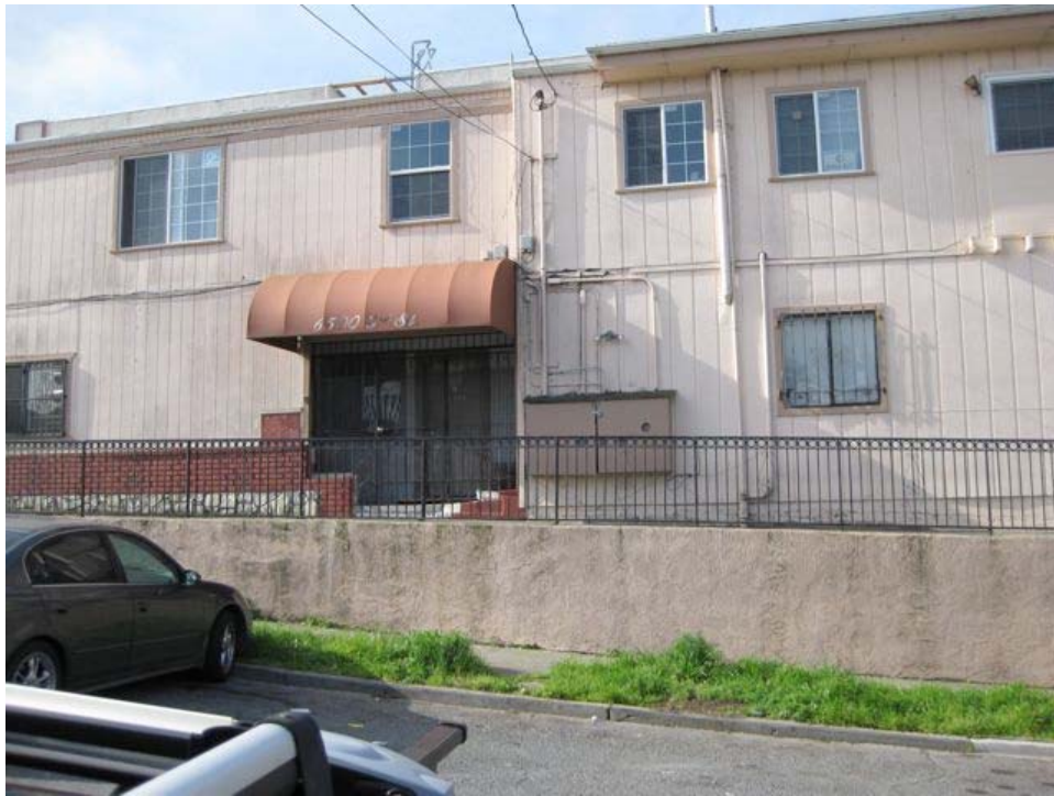
3 rd Street and Key Avenue: deteriorated siding, overgrown landscaping.
