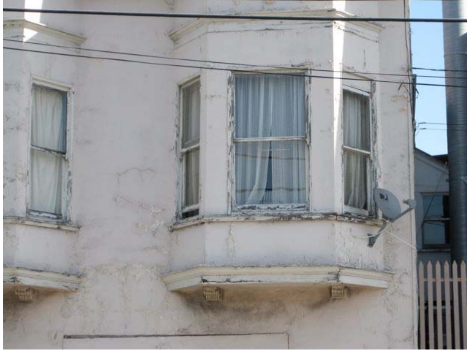
McKinnon Avenue near Newhall Street (close up of above): cracked wall, dry rot, peeling paint.
