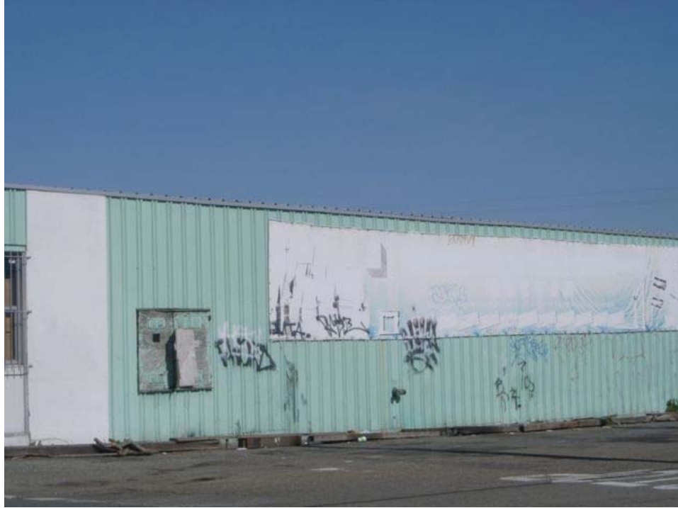
Oakdale Avenue near Rankin Street: graffiti, deteriorated sign, boarded windows.
