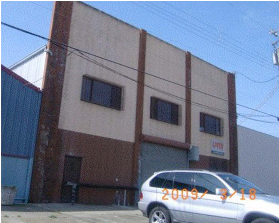
Donner Avenue between Jennings Street and Ingalls Street: deteriorated façade, peeling paint.
