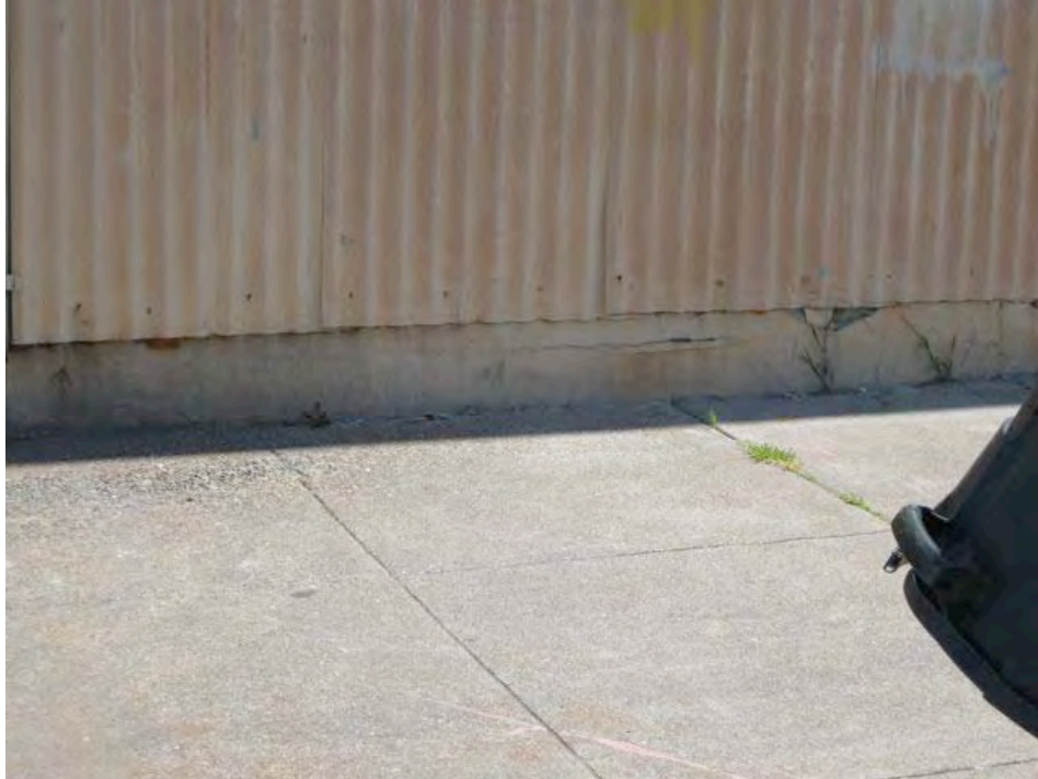
Kirkwood Avenue near Rankin Street: cracked foundation.
