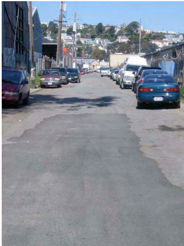
Newcomb Avenue near I-280: lack of sidewalks and deteriorated pavement.
