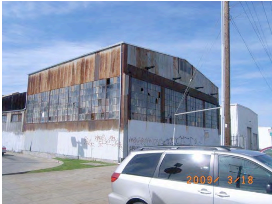
Bayshore Boulevard near Costa Street: extensive deterioration, broken windows, deteriorated siding, graffiti, eroded foundation.
