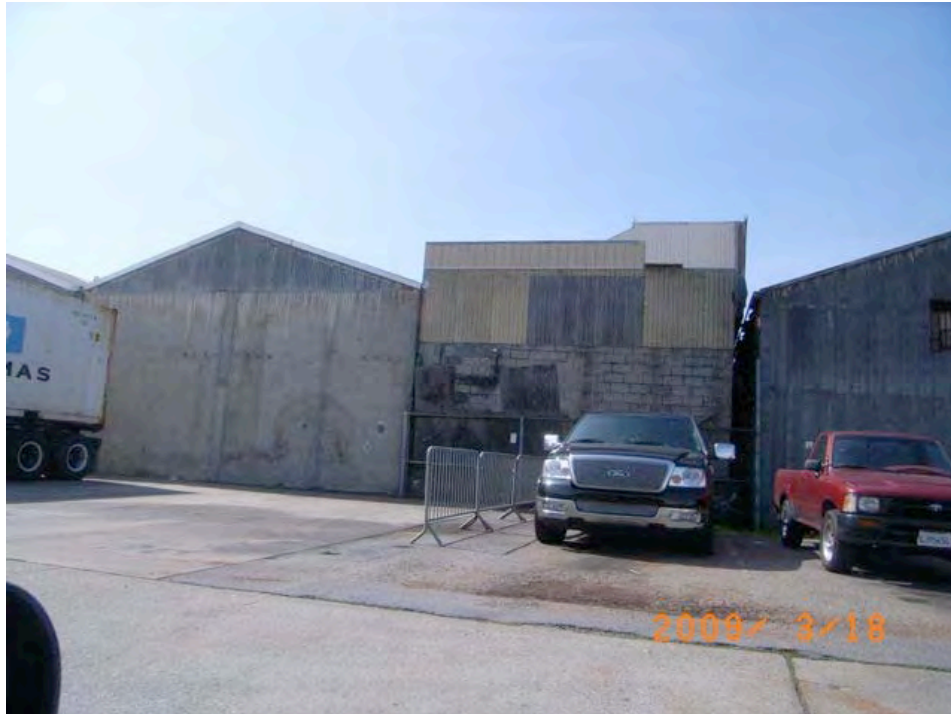
Donner Avenue between 3 rd Street and Jennings Street: damaged siding, informal and substandard construction.
