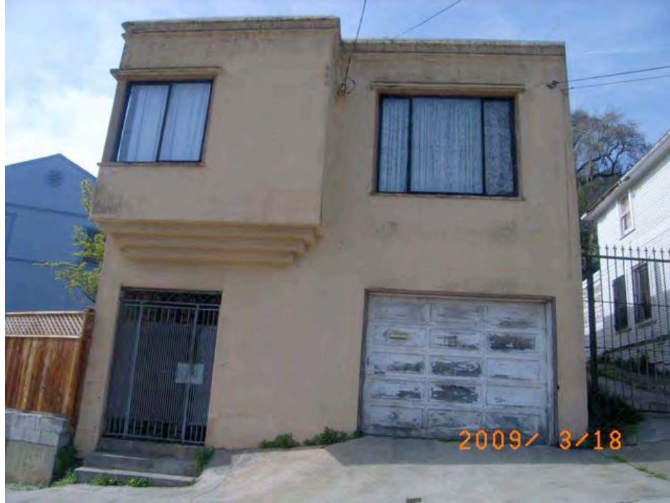
Ignacio Avenue near Ingerson Avenue: cracked wall, peeling paint, water damage, extensive deterioration.
