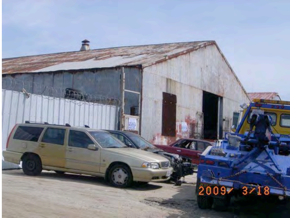
Underwood Avenue near Ingalls Street: deteriorated and rusted roofing and siding, razor wire security fence.
