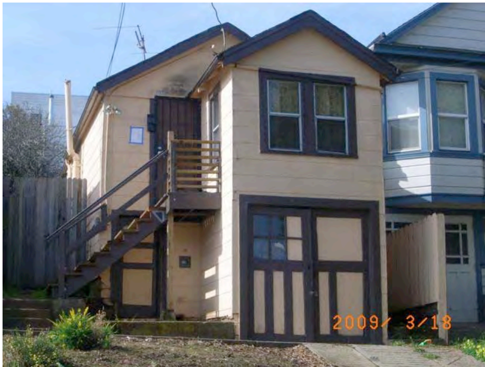
Ingerson Avenue near Ingalls Street: smoke damage above door, broken/missing eaves.
