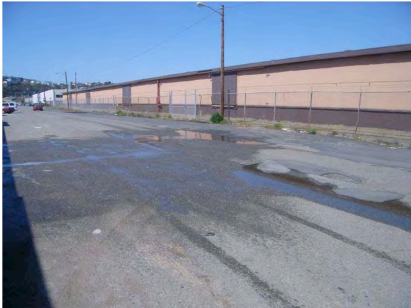
McKinnon Avenue near I-280: standing water, deteriorated pavement.
