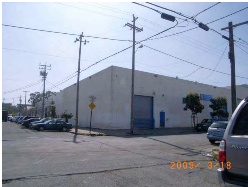
Donner Avenue near Ingalls Street: faded paint, partially reinforced masonry.
