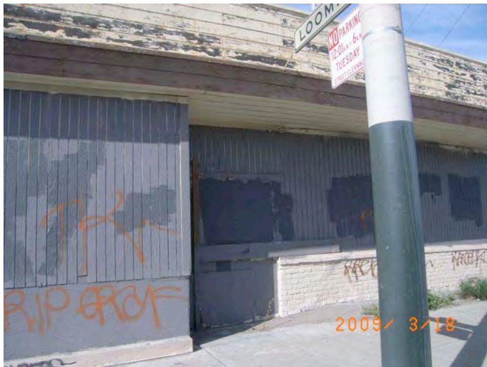
Industrial Street near Loomis Street (close up of above): vacant and dilapidated building, peeling paint, dry rot, graffiti.
