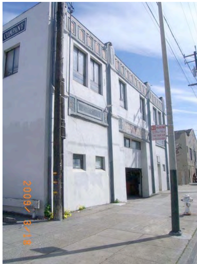
Bayshore Boulevard near Costa Street: peeling paint and cracked wall.
