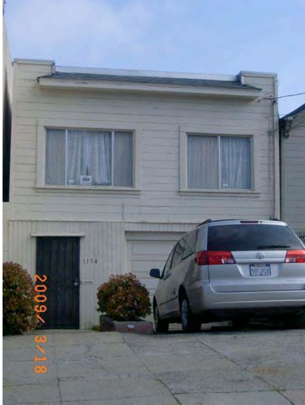
Gilman Avenue near Ingalls Street: peeling paint, deteriorated eaves, cracked sidewalk.
