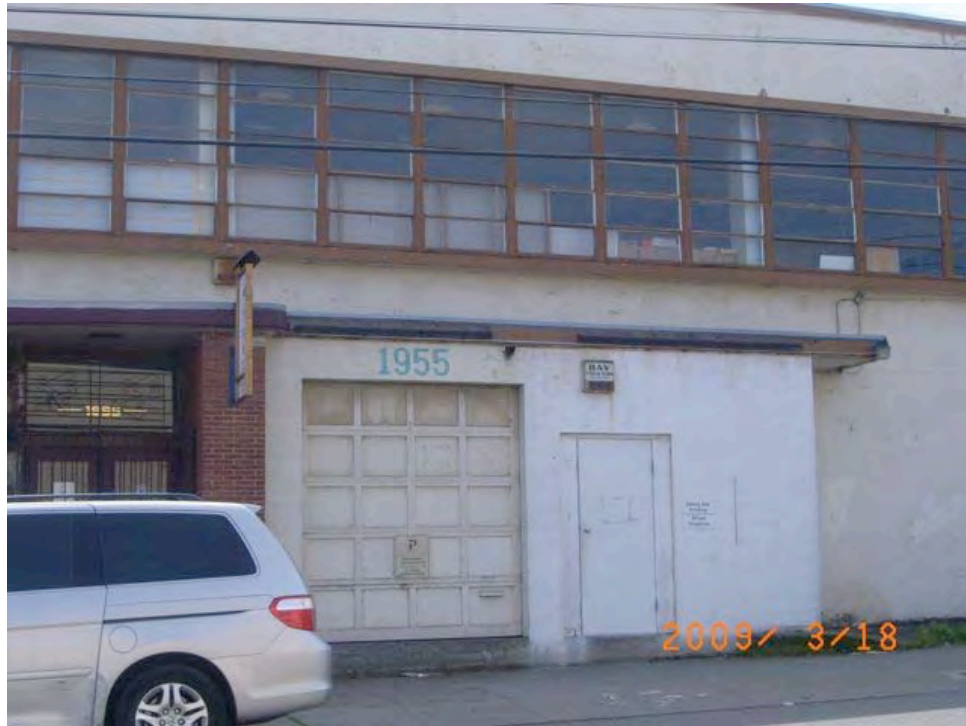
Carroll Avenue near Phelps Street: peeling paint, cracked siding, deterioration.
