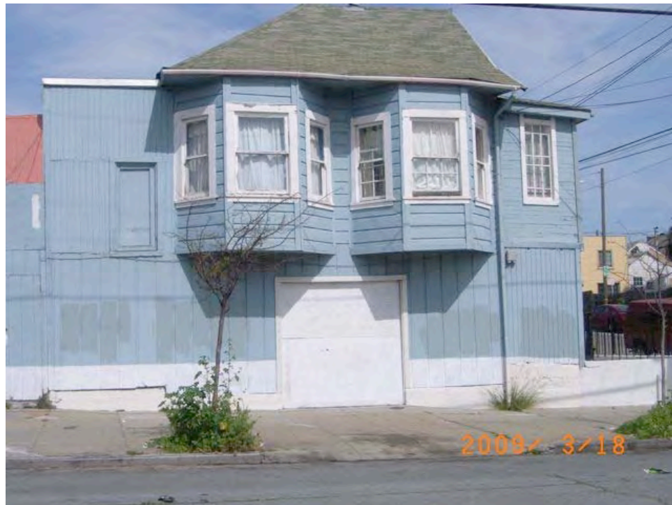
Van Dyke Avenue near Keith Street: damaged wood siding, sagging roof, cracked foundation.
