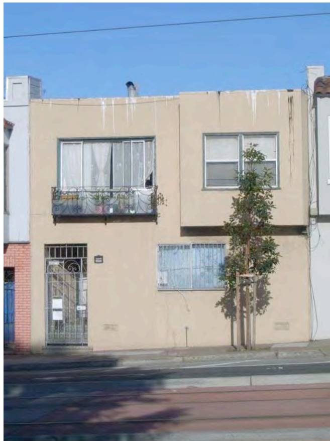
3 rd Street near Yosemite Avenue: deteriorated building, exposed wiring, water damage, cracked wall.
