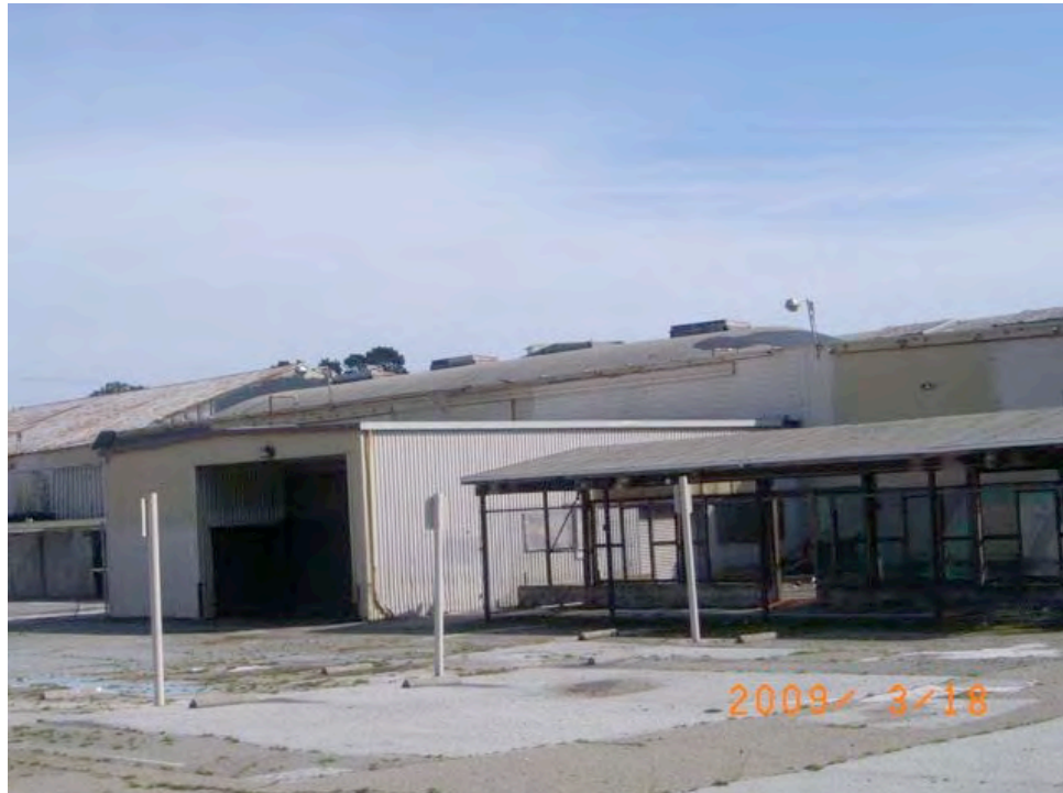
Bayshore Boulevard near Cortland Avenue: rusted roof, peeling paint, dilapidated pavement, extensive deterioration.
