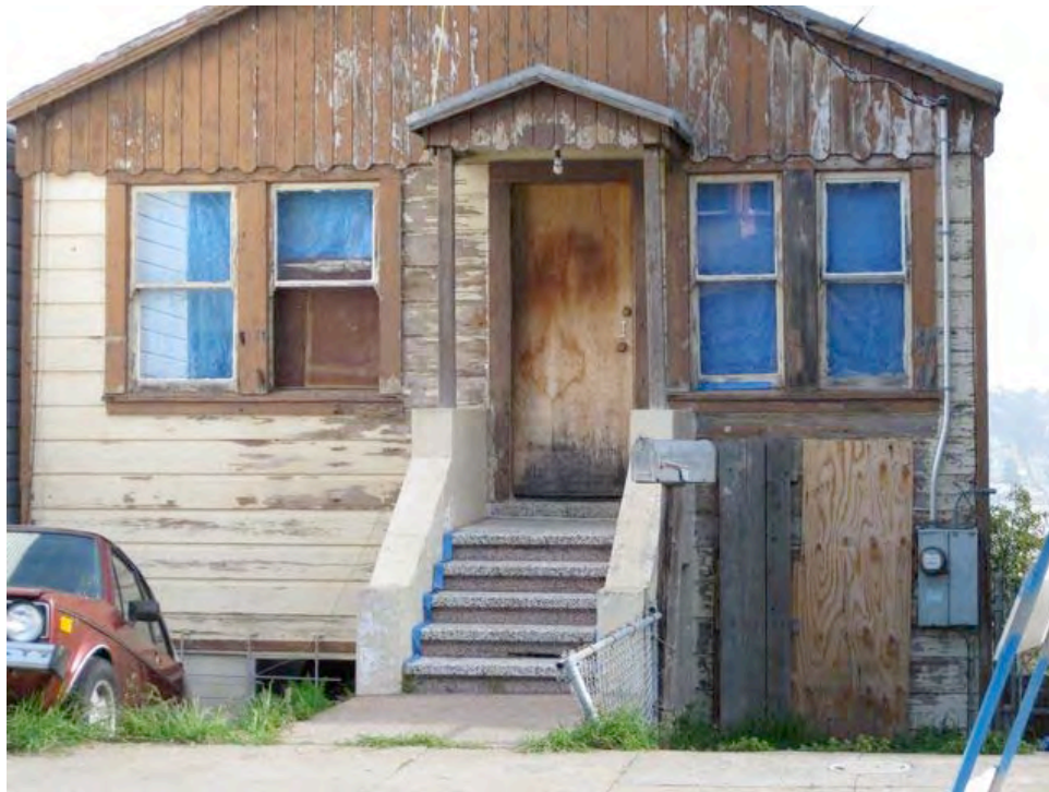
Jamestown Avenue near Ingalls Street: apparently abandoned dilapidated building, informal and substandard construction, peeling paint, broken and boarded windows, overgrown landscaping, abandoned vehicle.
