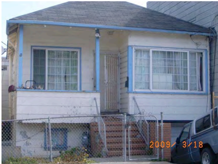
Hollister Avenue near Hawes Street: deterioration, peeling/cracking siding, peeling paint, external wiring.
