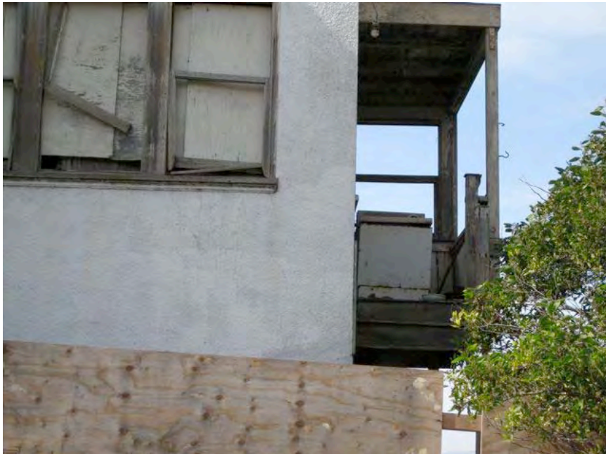
Newcomb Avenue near Lane Street: abandoned house, boarded windows, dry rot, outdoor storage, cracked wall, informal and substandard construction.
