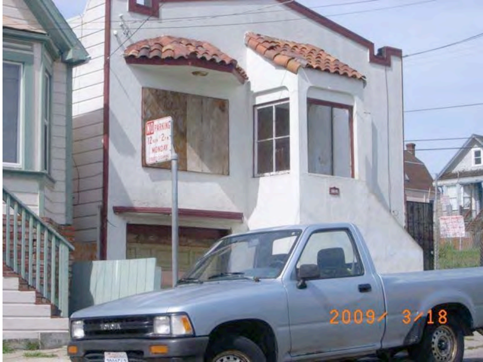
Keith Street near Underwood Avenue: vacant property with no broker information, boarded windows, roof deterioration, evidence of dry rot.
