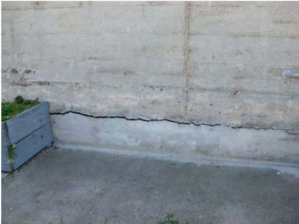
Toland Street near Galvez Avenue: cracked foundation.
