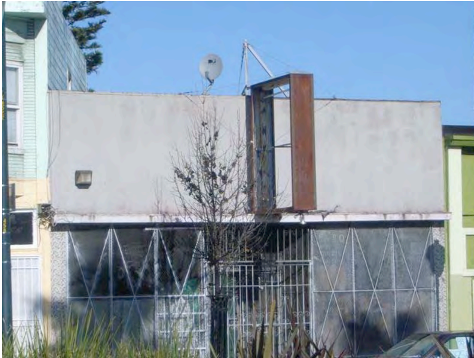
3 rd Street near LaSalle Avenue: vacant business space, dilapidated signage, water damage, peeling paint, deterioration.
