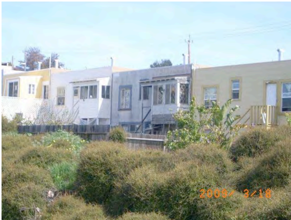
Reddy Street near Williams Avenue, rear of home: deferred maintenance, peeling paint.
