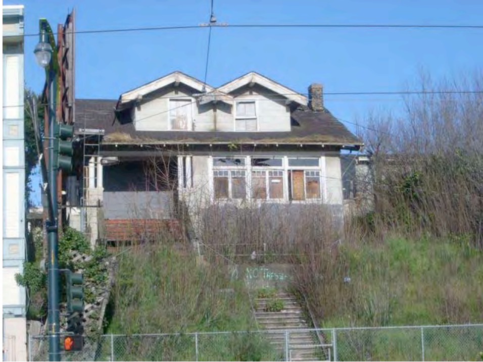
3 rd Street near Williams Avenue: extensive dilapidation, deteriorating roofing, broken and boarded windows, overgrown landscaping.
