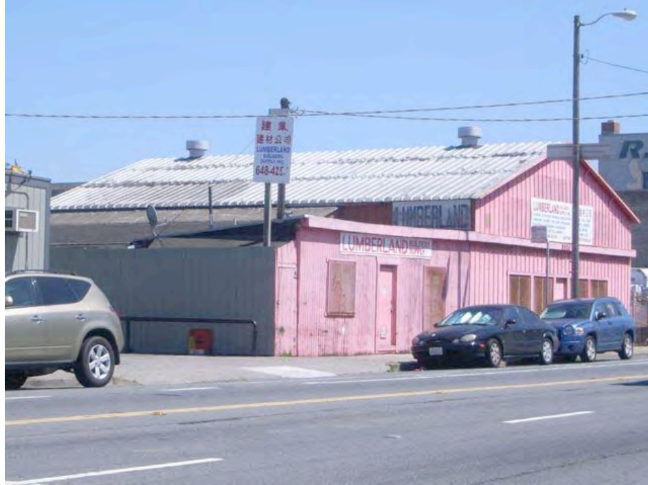
Oakdale Avenue near Barneveld Avenue: vacant business space, boarded windows, substandard and informal construction, peeling paint, graffiti, deteriorating and sagging roof.
