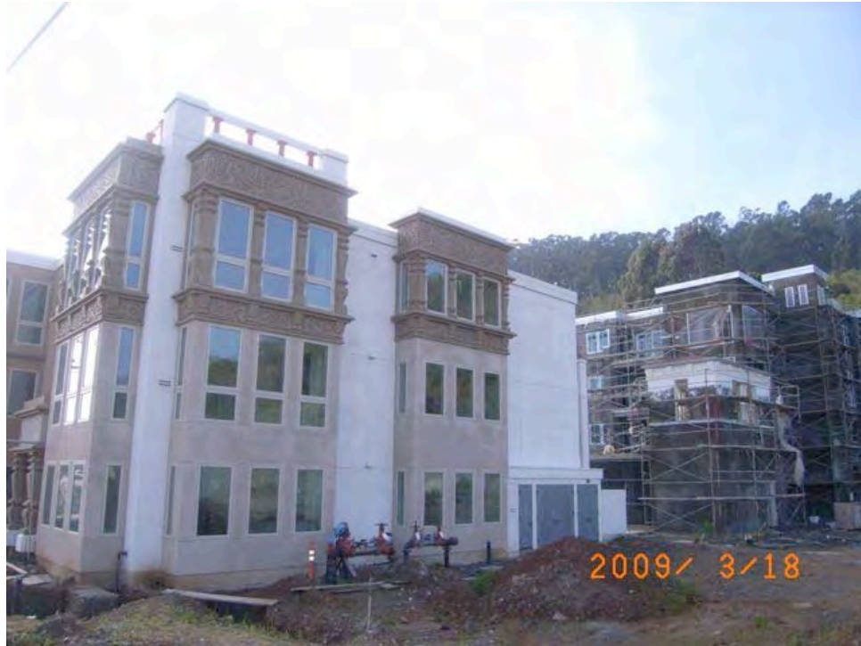
Jamestown Avenue near Redondo Street: suspended residential development.
