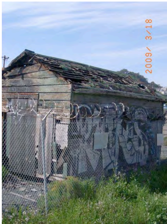
Indiana Street near Tulare Street: uninhabitable dilapidated building, collapsed roof, dry rot, peeling paint, graffiti.
