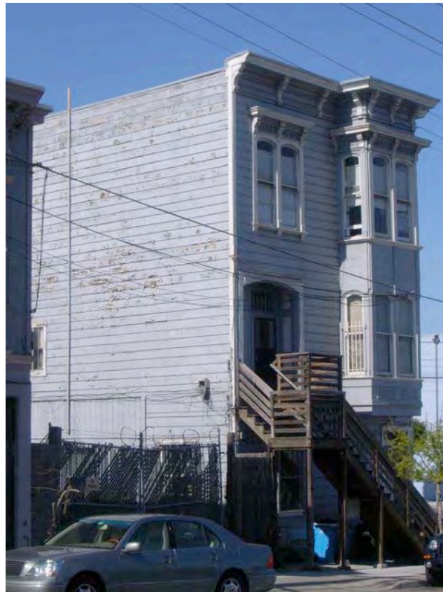
Oakdale Avenue near Quint Street: deteriorated building, dry rot, peeling paint.
