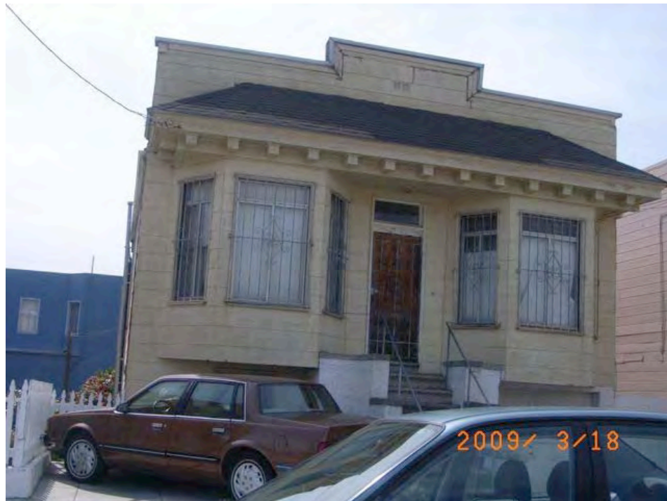
Underwood Avenue at Jennings Street: chipped/cracked siding, security grates and door, evidence of dry rot, deferred maintenance.
