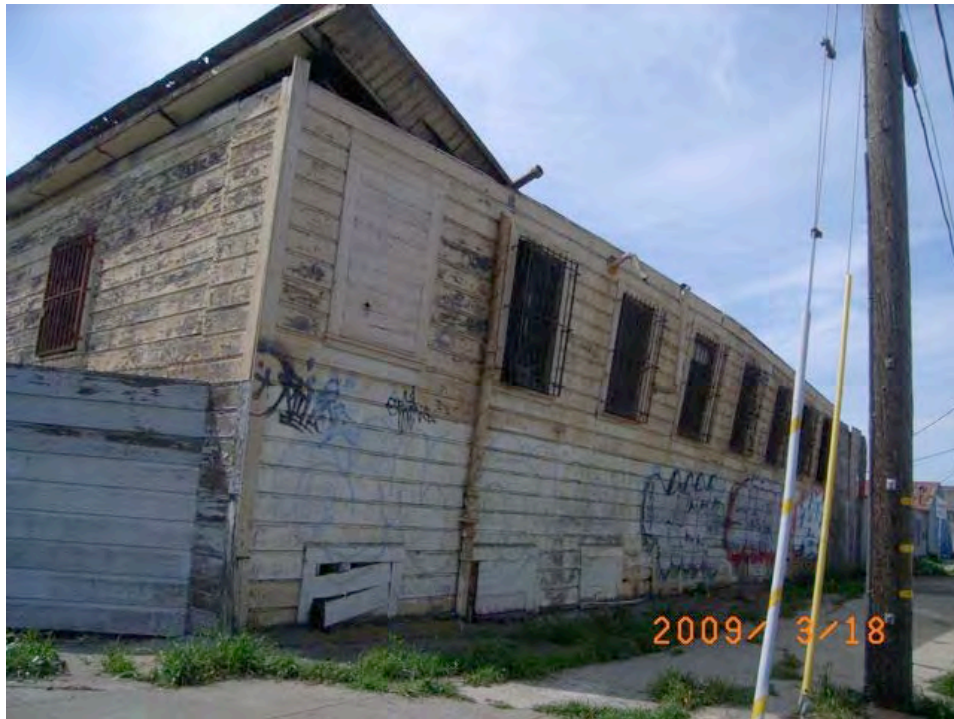
Thomas Avenue near Hawes Street: wall collapsing onto a public right-of-way, graffiti, peeling paint, rotting wood, deteriorated and overgrown sidewalk.
