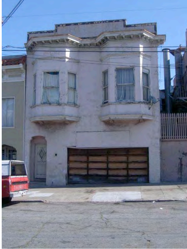
McKinnon Avenue near Newhall Street: extensive deferred maintenance, sagging floor above garage, cracked wall, dry rot, broken windows.
