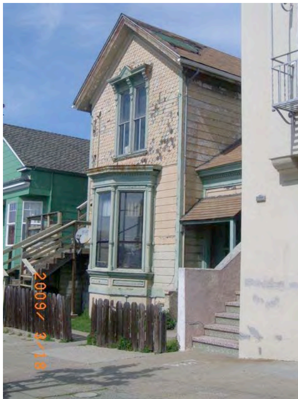
Palou Avenue near Lane Street: peeling paint, rotting wood, dilapidated roof, water damage.
