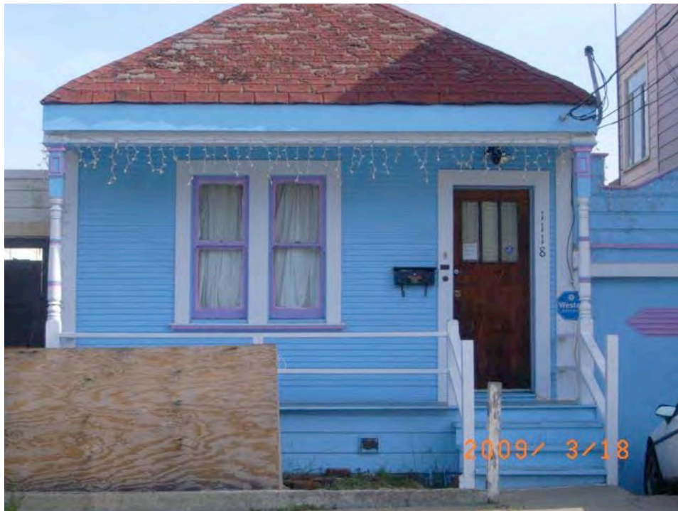
Hollister Avenue near Ingalls Street: dilapidated roofing, deteriorated garage siding.
