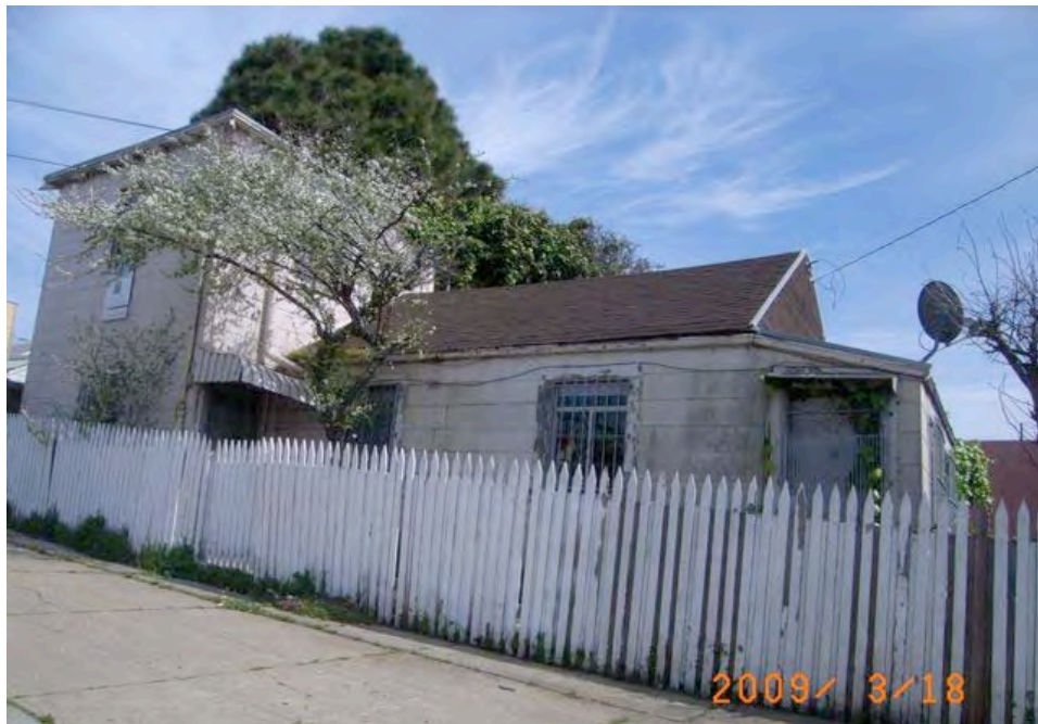
Keith Street near Underwood Avenue (different angle on property above): sagging roof, dry rot, deteriorated windows, deteriorated fence, external wiring, extensive deterioration.
