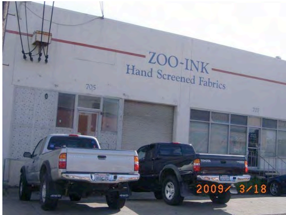
Cesar Chavez Street near Michigan Street: large crack on wall above door, peeling paint.
