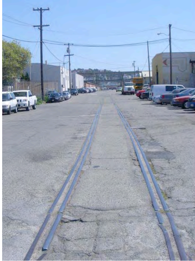
McKinnon Avenue near Barneveld Avenue: cracked pavement, abandoned rail line, lack of sidewalks.
