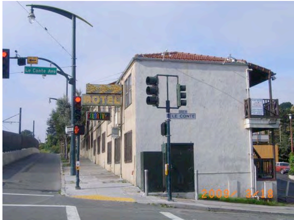
LeConte Avenue and 3 rd Street: motel property for sale exhibiting faded and peeling paint, cracked walls, extensive deferred maintenance, protective bars on windows.
