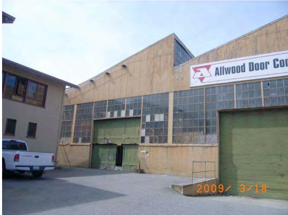
3 rd Street near Egbert Avenue: extensive deterioration rusted metal siding, peeling paint, broken windows.
