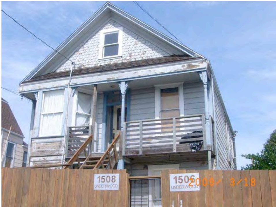
Underwood Avenue near Keith Street: deterioration, informal and substandard construction, peeling paint, evidence of dry rot.
