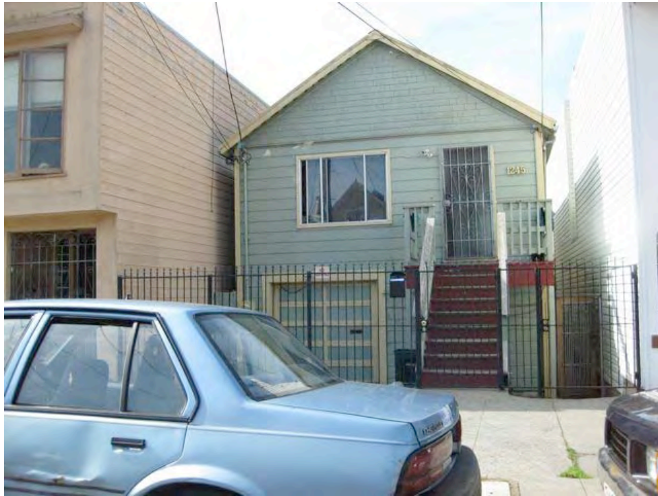
Hollister Avenue near Jennings Street: peeling and faded paint.
