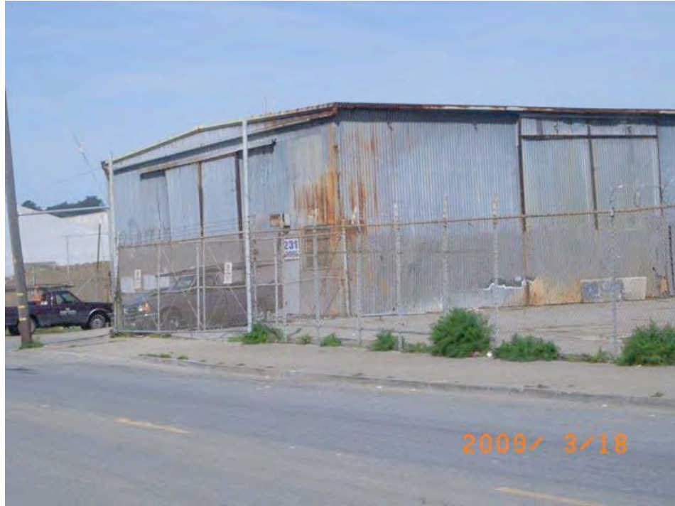
Loomis Street near Waterloo Street: rusted and dilapidated roofing and siding, razor wire security fencing.
