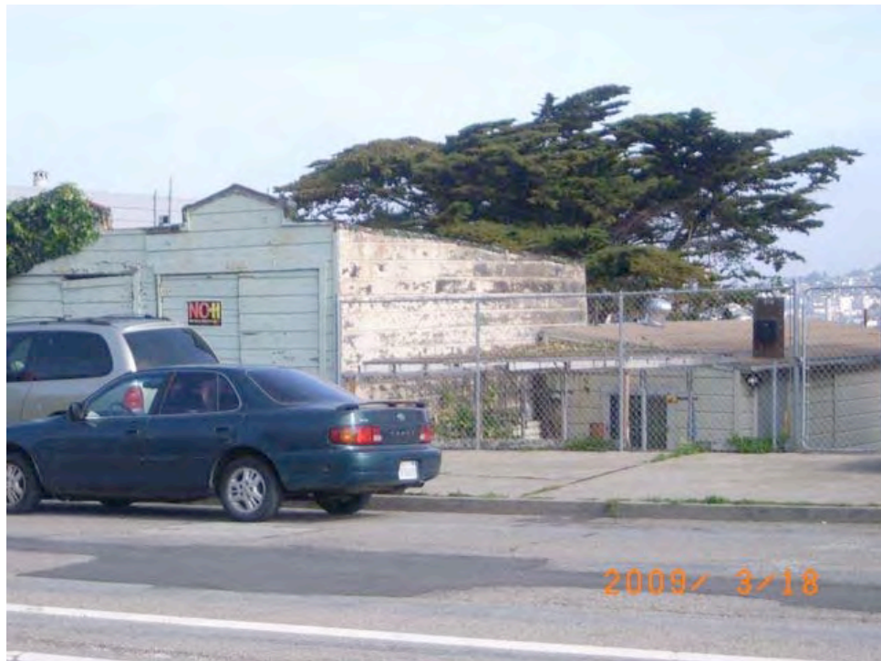
Jamestown Avenue near Hawes Street: peeling paint, water damage, alignment problems, extensive deterioration.
