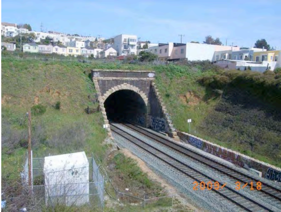
Williams Avenue: trash accumulation, graffiti near rail tunnel.
