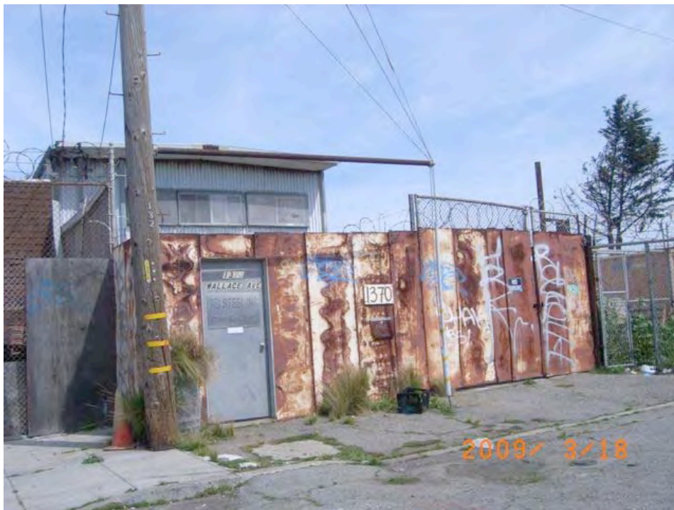
Wallace Avenue near Ingalls Street: informal and substandard construction, deteriorated sidewalk, extensive deferred maintenance, razor wire security fence, rusted gate.
