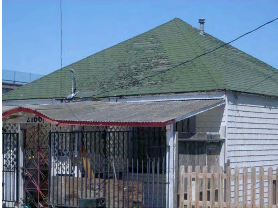
Revere Avenue near I-280: dilapidated building, dry rot deteriorating roofing, informal and substandard construction.
