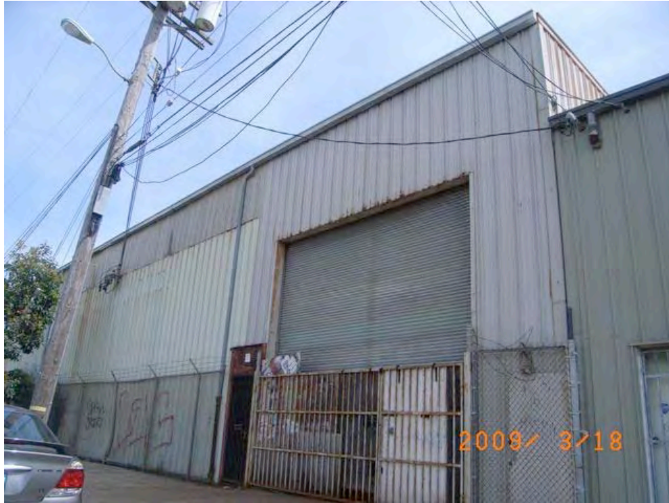
Ingalls Street near Bancroft Avenue: rusted and deteriorated siding, graffiti, security grate and barbed wire.
