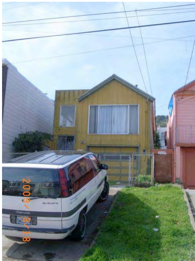
Hollister Avenue near Ingalls Street: security door, water-damaged siding, older windows.
