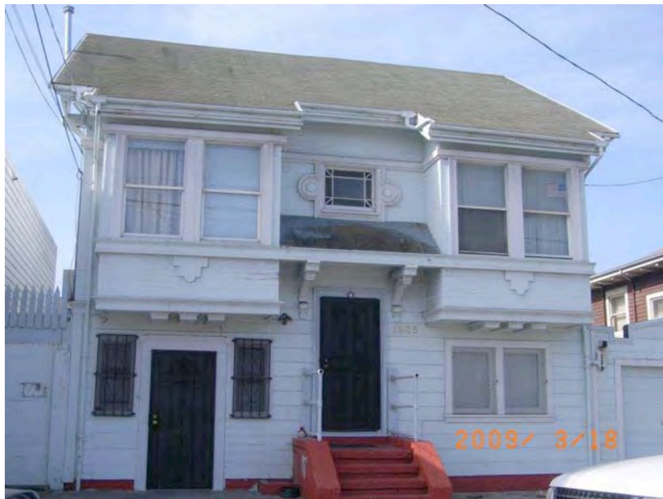
Hollister Avenue near Jennings Street: deteriorated roof, water damage, security door, window grates.
