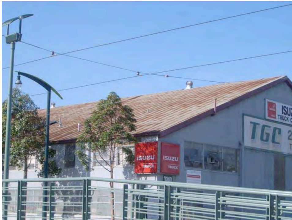
3rd Avenue near Tulare Street: roof rust and deterioration.
