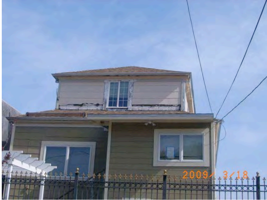
Fitzgerald Avenue near Hawes Street: extensive deterioration, dilapidated siding, evidence of serious dry rot.
