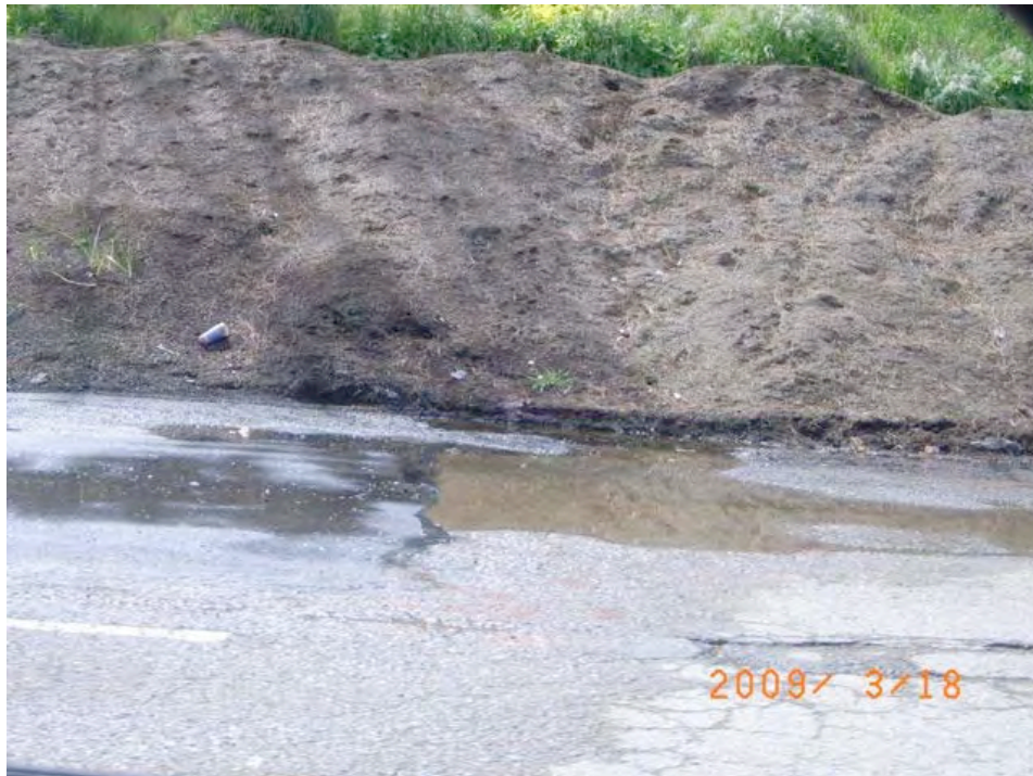
Carroll Avenue near Arelious Walker Drive (close up of above): standing water; lack of sidewalk, curb or gutters; and eroding hillside.
