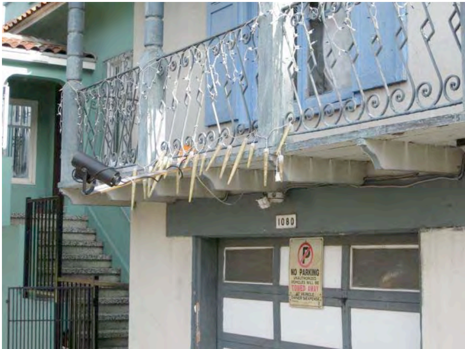
Key Avenue near 3 rd Street: security camera in front of garage, peeling paint.
