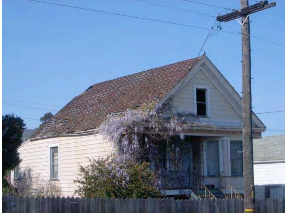
Oakdale Avenue near Quint Street: severely dilapidated building, sagging roof with large gaps, dry rot, broken windows.
