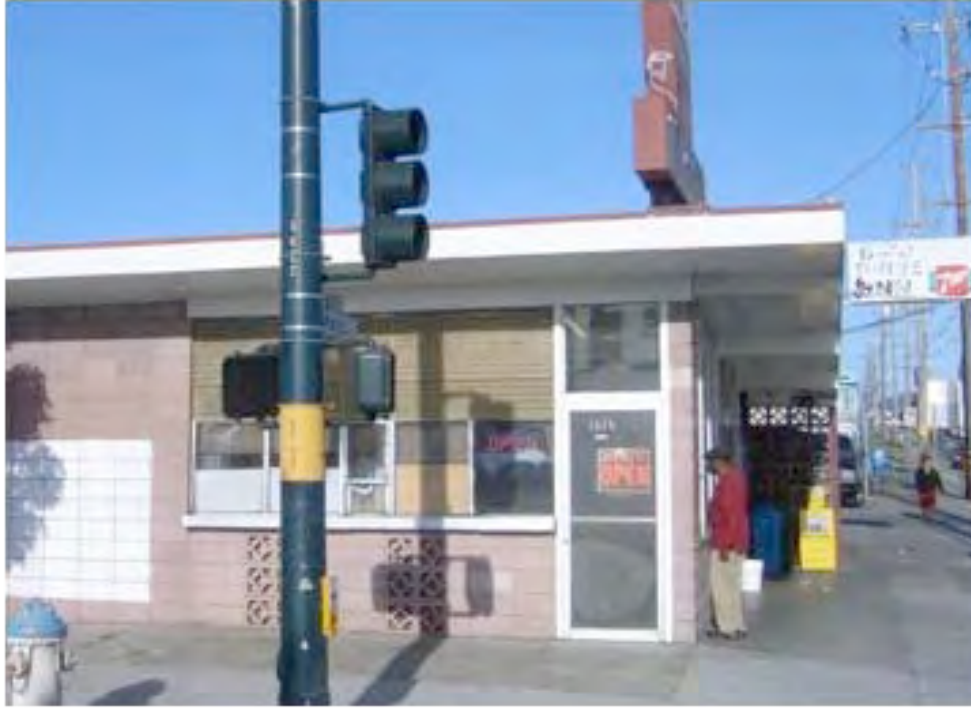
3 rd Street at Paul Avenue: deferred maintenance, graffiti on both signs, deteriorated signage.
