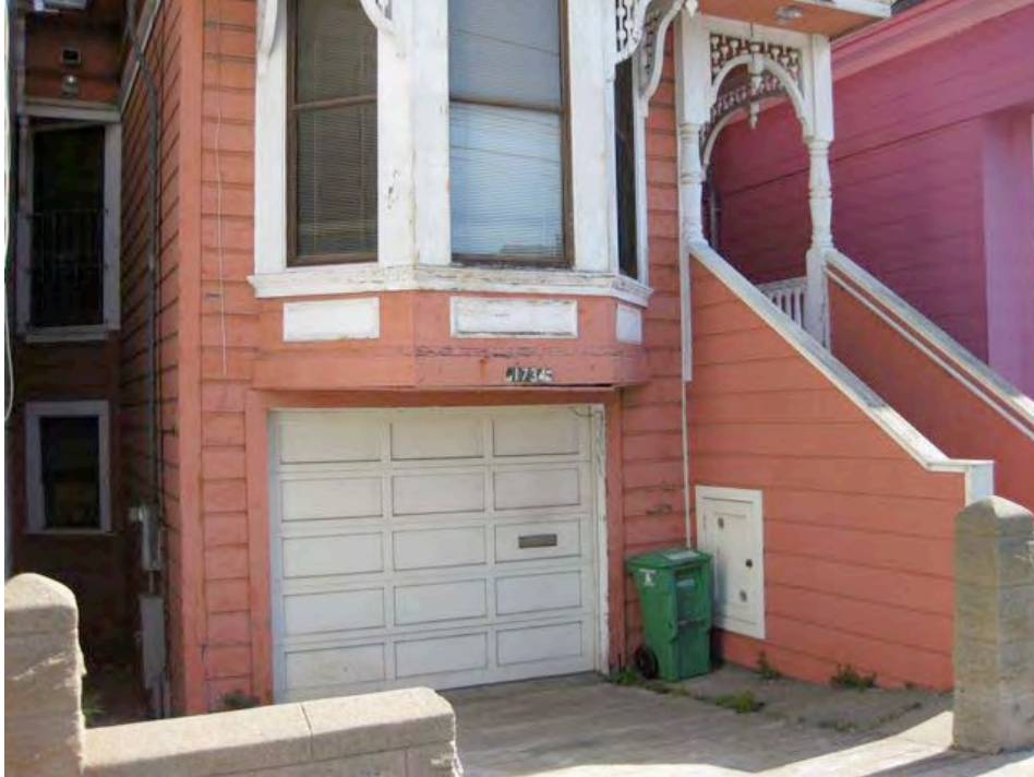
Newcomb Avenue near Newhall Street (close up of above): extensive deterioration, peeling paint, rotting wood, and deteriorating siding.
