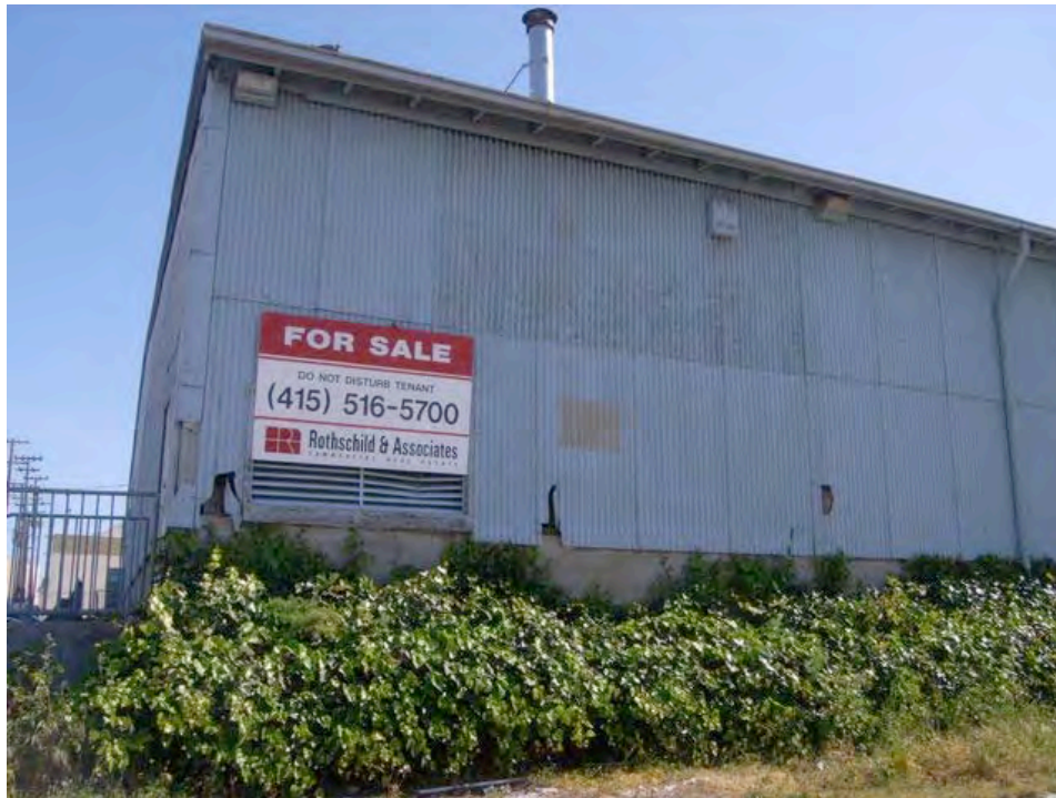
Toland Street near Galvez Avenue: deteriorated siding, extensive deterioration.
