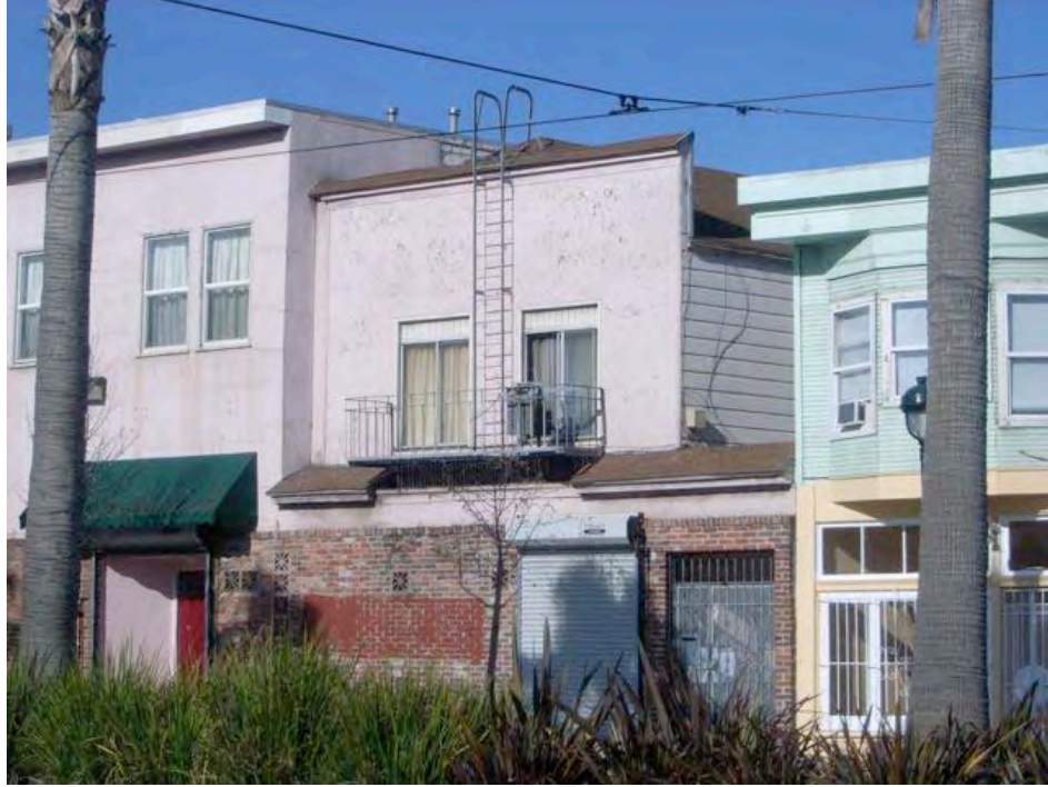
3 rd Street near LaSalle Avenue: peeling paint, deferred maintenance, deteriorating roofing.
