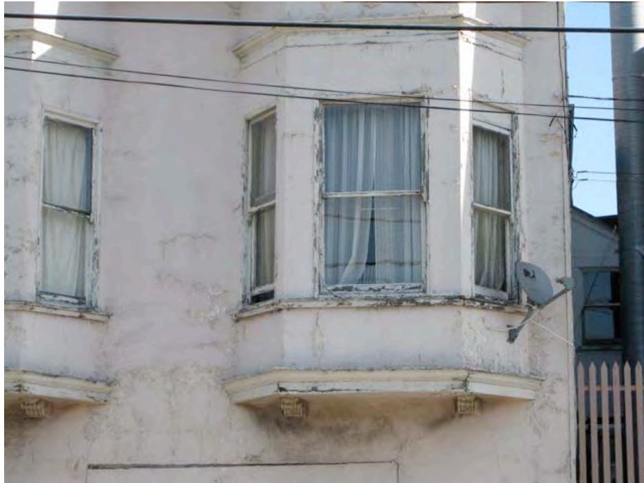
McKinnon Avenue near Newhall Street (close up of above): cracked wall, dry rot, peeling paint.
