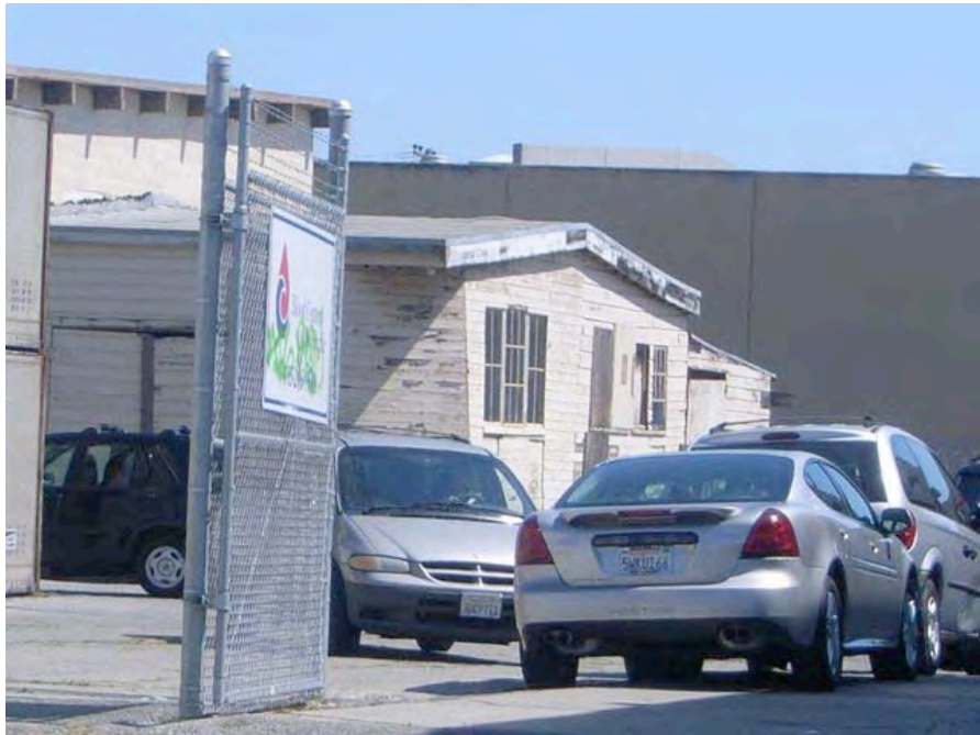
Barneveld Avenue near McKinnon Avenue: peeling paint, extensive dilapidation, alignment issues.
