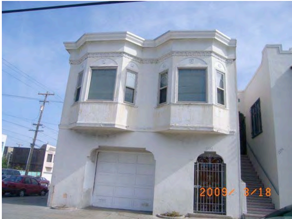
Gilman Avenue near Jennings Street: peeling paint, water damage, deferred maintenance.
