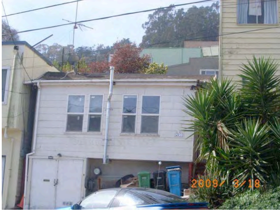
Ignacio Avenue near Ingerson Avenue: informal and substandard construction, sagging roof, alignment problems, faded paint.
