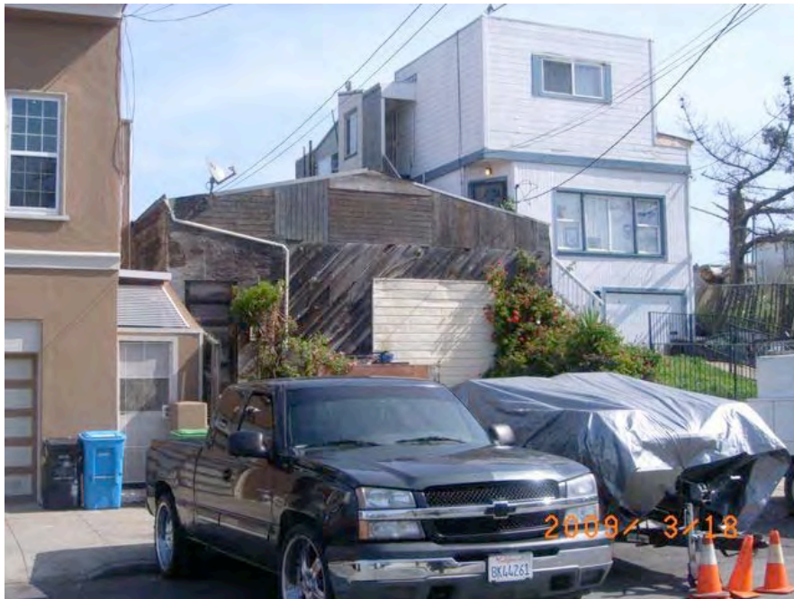
Egbert Avenue near Hawes Street: informal and substandard construction, water damage to wood siding.
