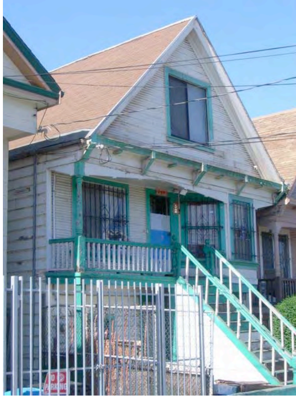
Kirkwood Avenue near Newhall Street: extensive deterioration, peeling paint, dry rot, informal and substandard construction, security bars.
