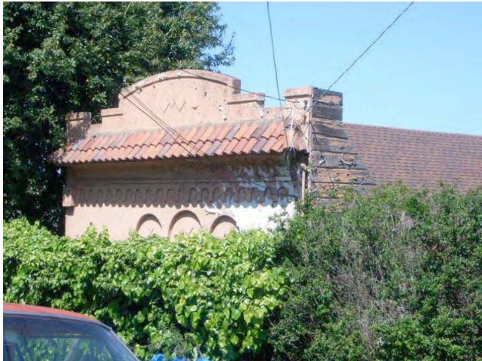
Revere Avenue near I-280: peeling paint, deferred maintenance.
