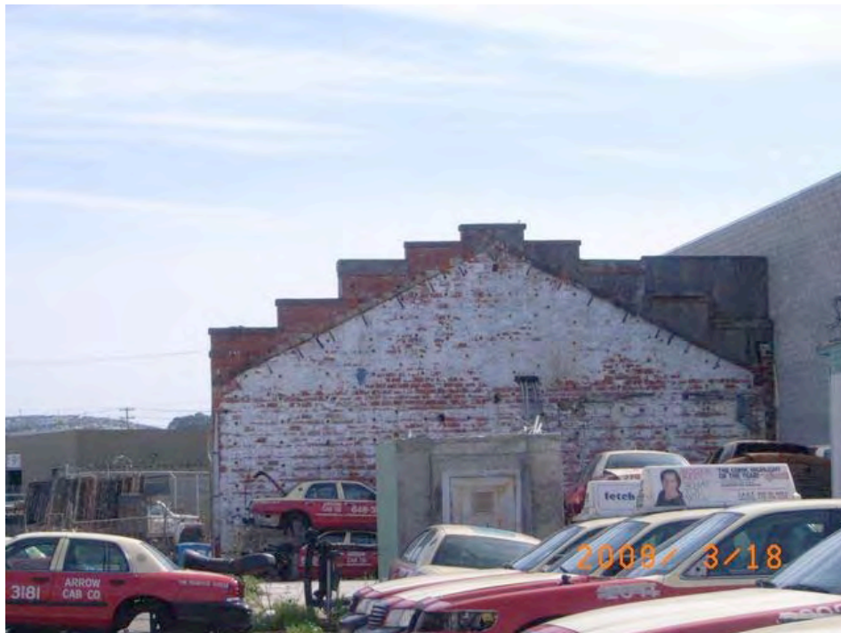
Marin Street near Jerrold Avenue: outdoor storage, unreinforced masonry construction, extensive deterioration.
