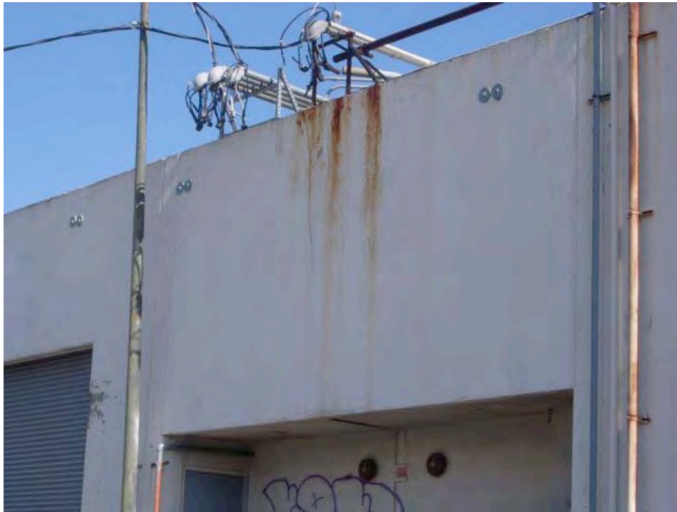
Newcomb Avenue near Rankin Street: cracked wall, water damage, peeling paint, graffiti.
