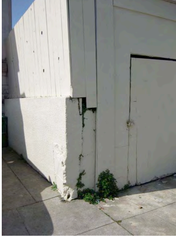
Egbert Avenue near Hawes Street: cracking foundation wall, rotting wood, alignment problems.
