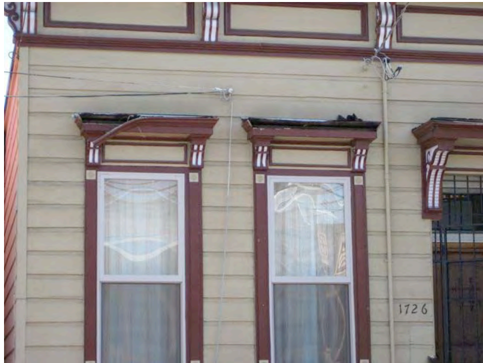
Newcomb Avenue near Newhall Street: dry rot and deteriorating siding.
