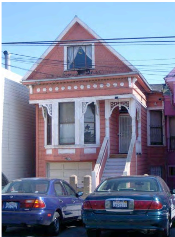
Newcomb Avenue near Newhall Street: cracked wall, peeling paint, evidence of dry rot.
