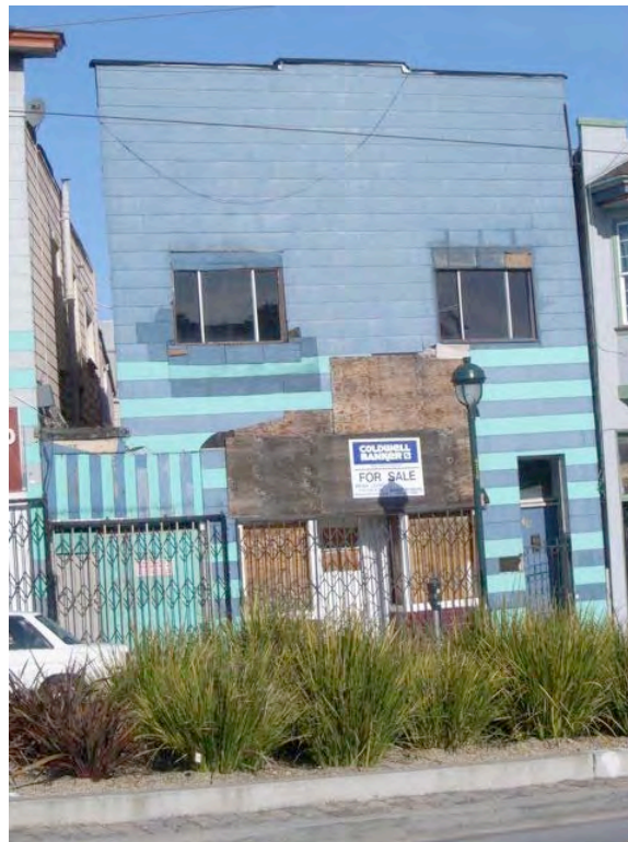
3 rd Street near Oakdale Avenue: informal and substandard construction, extensive dilapidation, missing siding, boarded windows and door, alignment problems, water damage.
