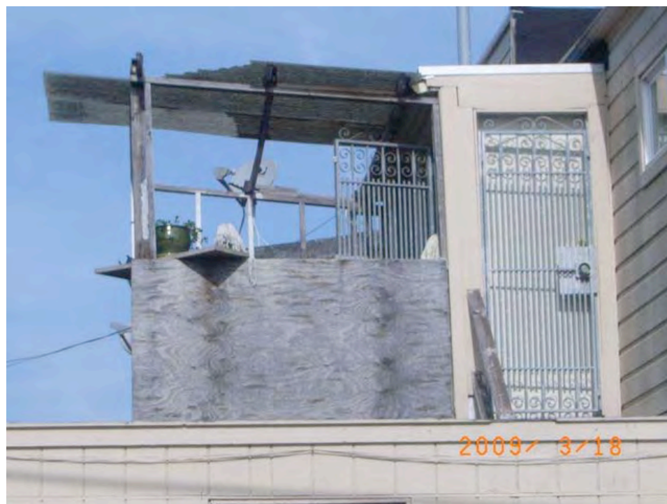
Jennings Street near Hollister Avenue: informal and substandard construction, deteriorated roofing, alignment problems.
