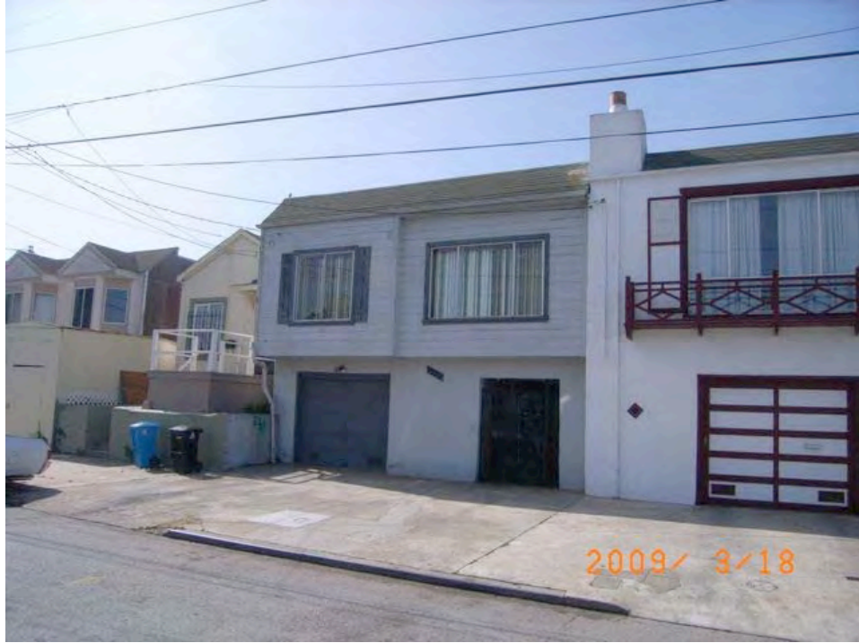
Egbert Avenue near Hawes Street: peeling paint, graffiti.
