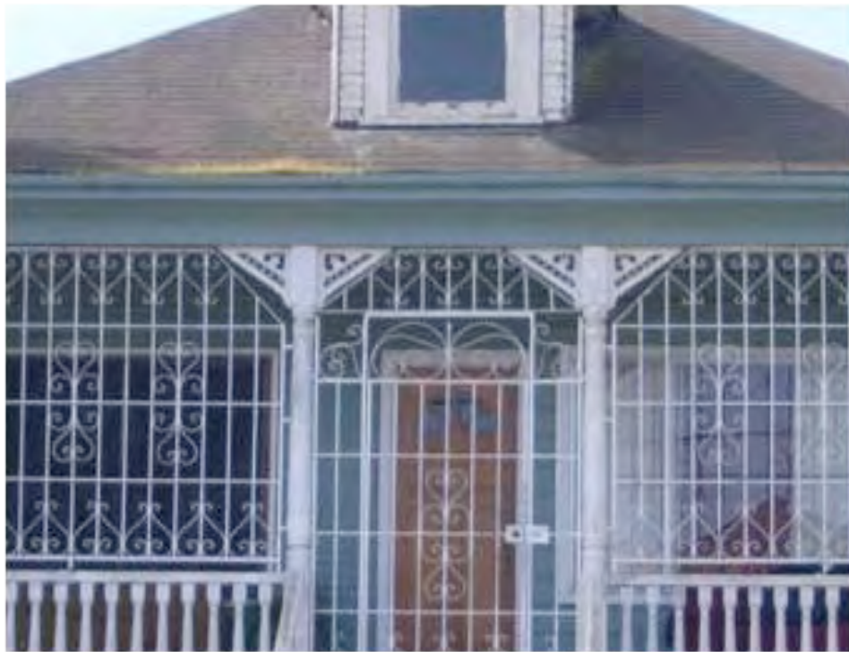
Hollister Avenue near Jennings Street (close up of above): vegetation growing from rain gutter, deteriorated attic window.
