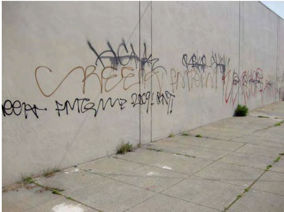
Carroll Avenue near Keith Street: deferred sidewalk maintenance, graffiti.
