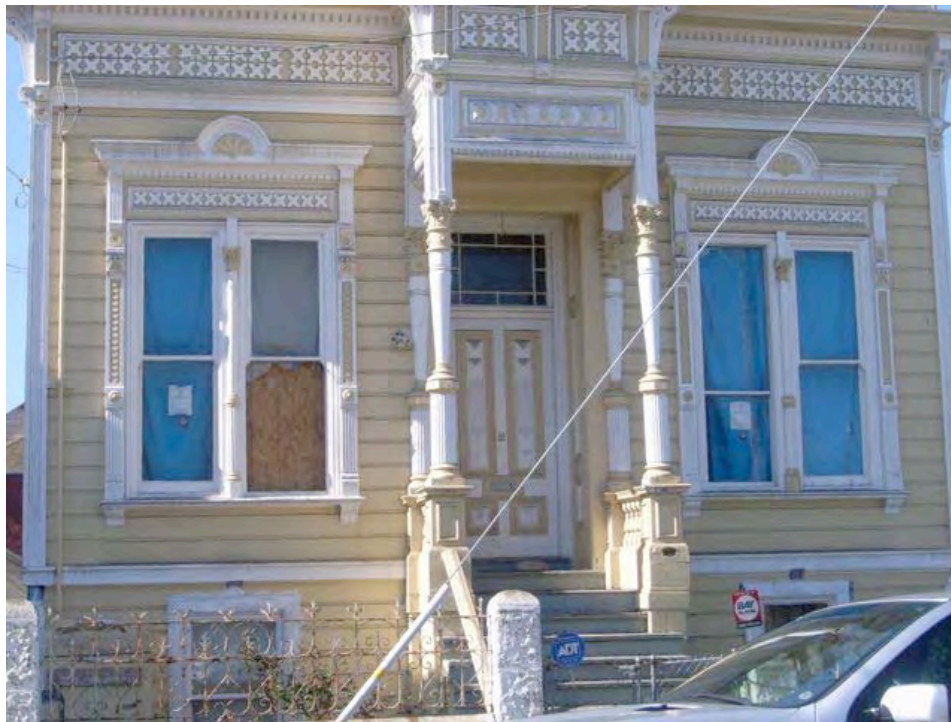
Jerrold Avenue near 3 rd Street: broken and boarded windows, peeling paint, extensive deterioration.
