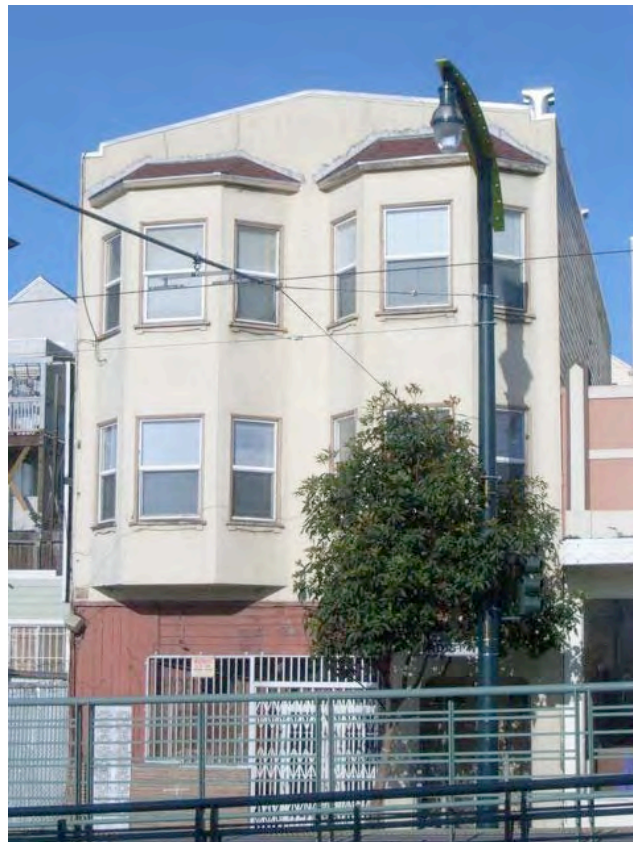
3 rd Street near Shafter Avenue: deteriorated siding, cracked wall, external wiring, peeling paint.
