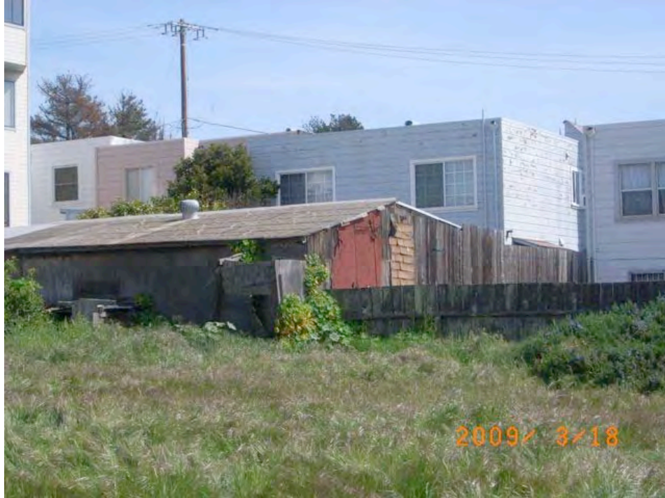
Reddy Street near Williams Avenue, rear of property: informal and substandard construction, peeling paint, deteriorated roofing.
