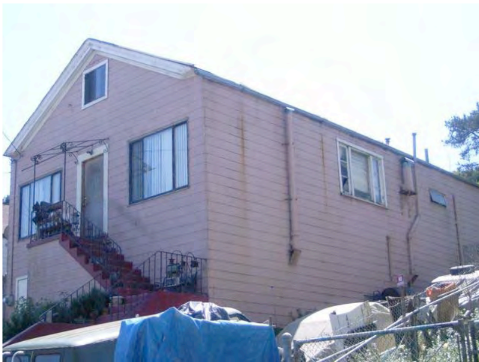
Revere Avenue near I-280: deferred maintenance, water damage on siding, possible dry rot.
