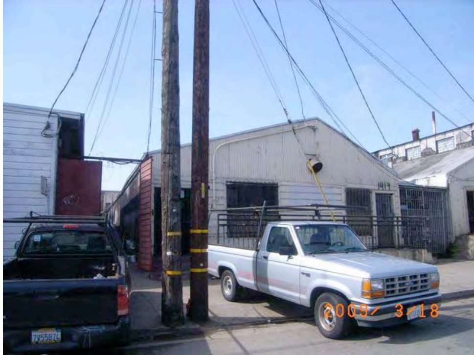
Egbert Avenue near Jennings Street: substandard exterior wiring, peeling paint, graffiti.
