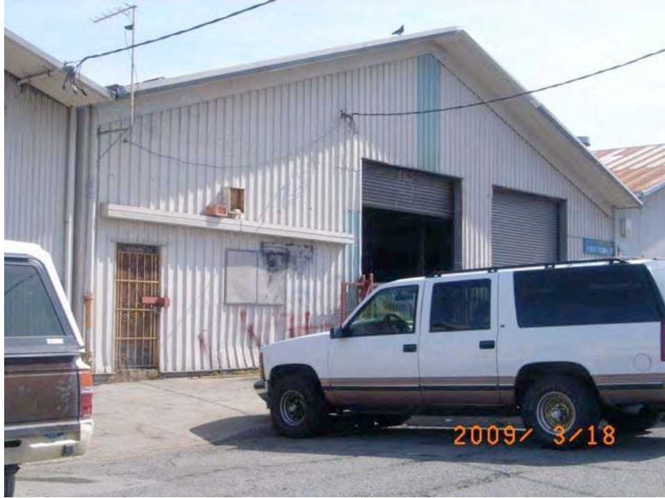
Donner Avenue near Ingalls Street: graffiti, deteriorated siding.
