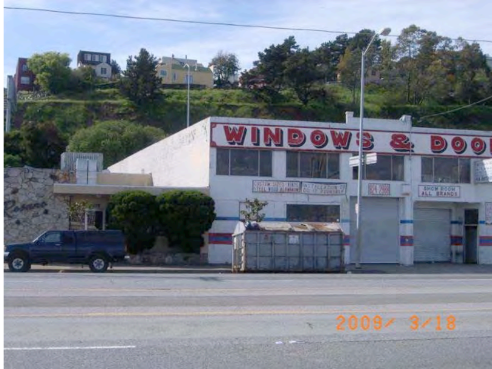
Bayshore Boulevard near Cortland Avenue: peeling paint, deteriorated signage.
