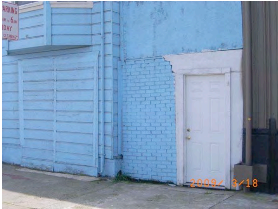
Egbert Avenue near Ingalls Street: informal and substandard construction, water damage, alignment problems.
