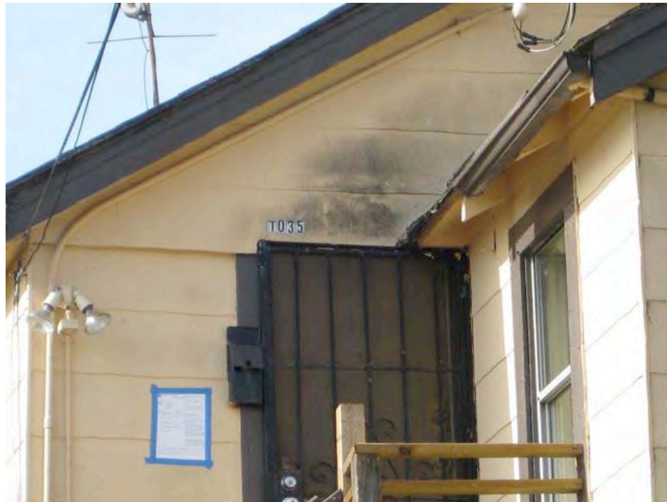
Ingerson Avenue near Ingalls Street (close up of above): smoke damage, broken/missing eave.
