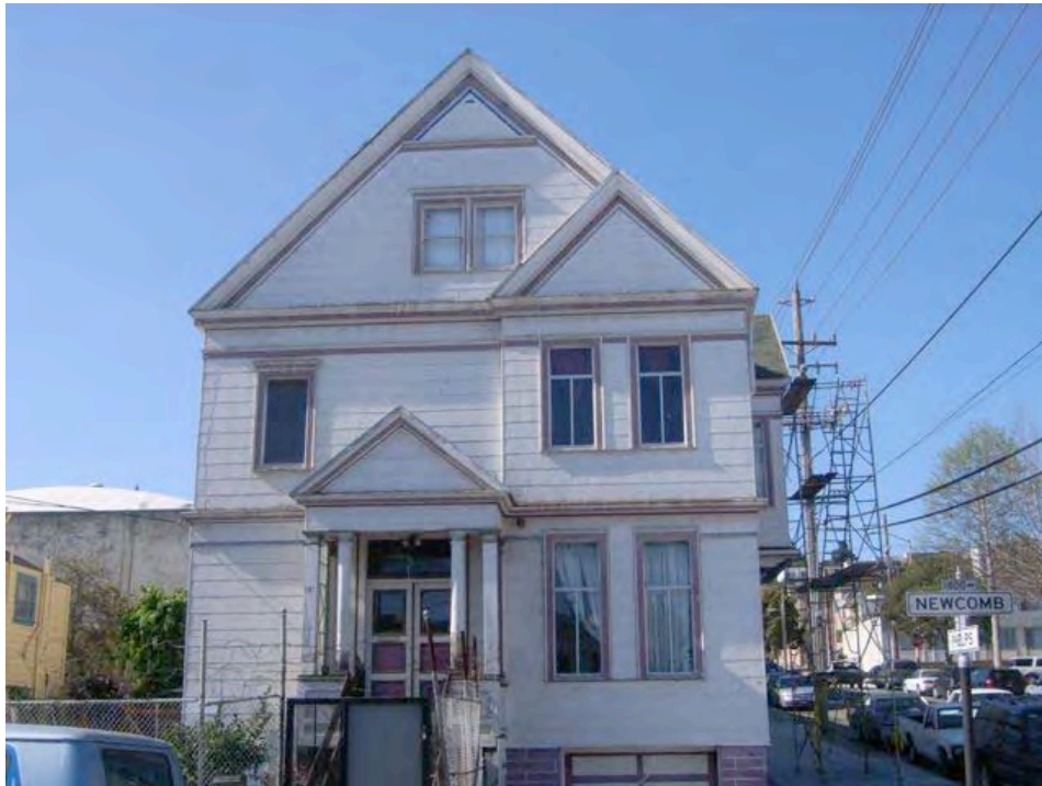
Newcomb Avenue at Phelps Street: external wiring, substandard and informal construction, peeling paint.
