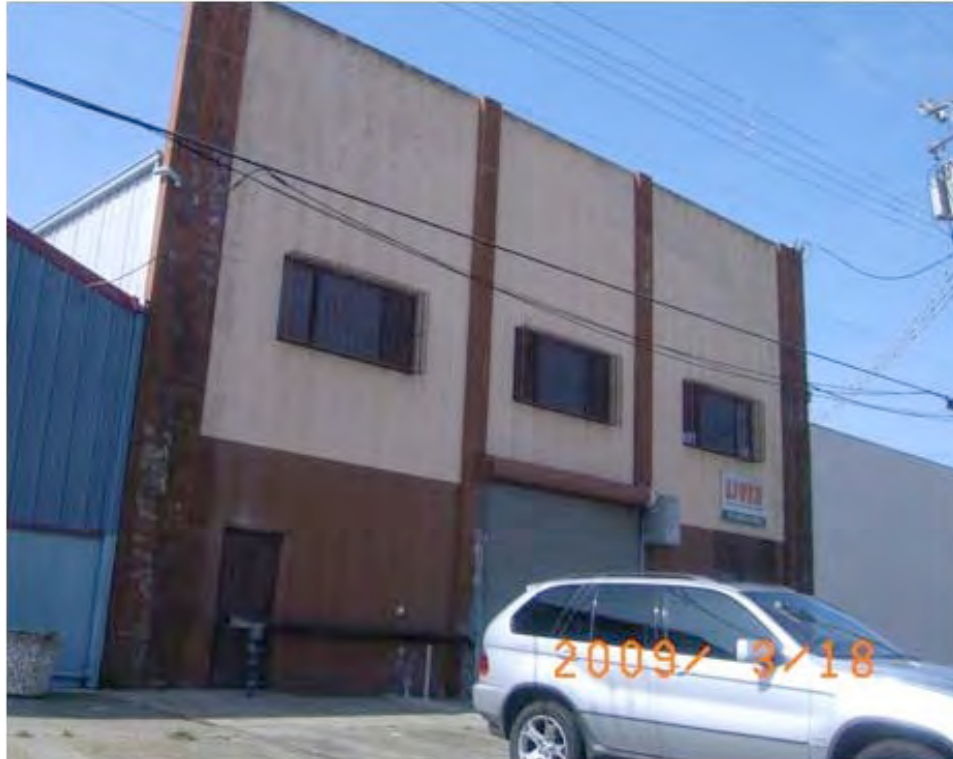
Donner Avenue between Jennings Street and Ingalls Street: deteriorated façade, peeling paint.
