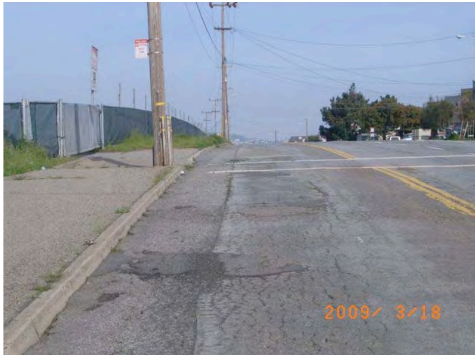
Jamestown Avenue near Ignacio Avenue: deteriorated pavement, cracked sidewalk, overgrown grass on sidewalk.
