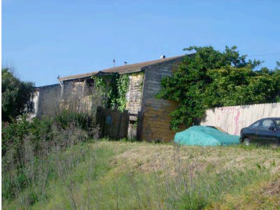
3 rd Street at Thornton Avenue: extensive deferred maintenance, peeling paint, graffiti, deteriorating roof and eaves,
