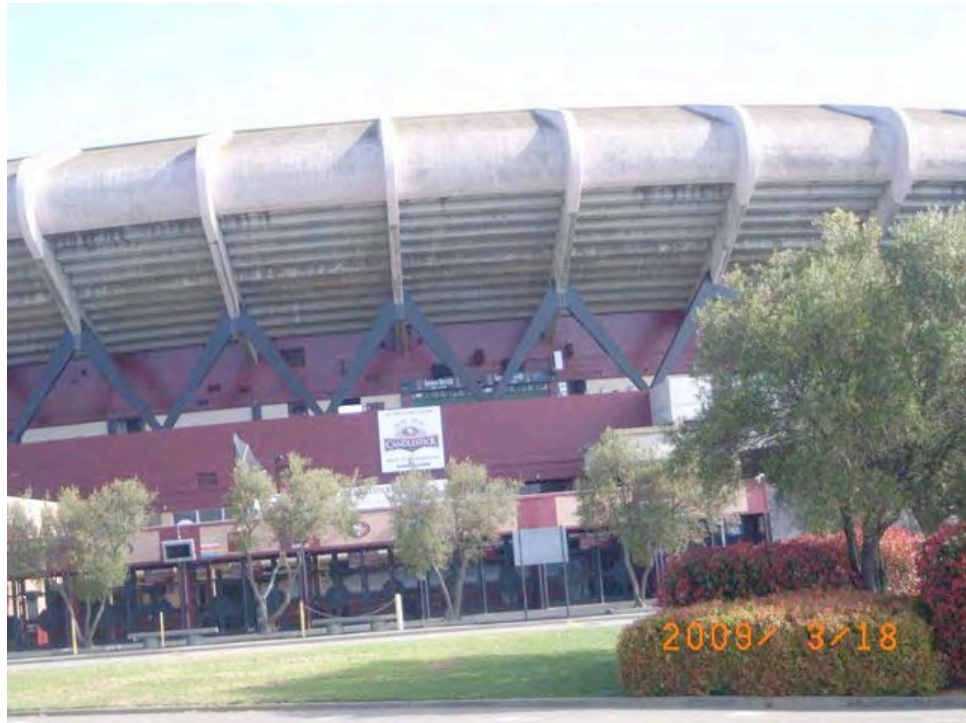
Jamestown Avenue: mold on Candlestick Stadium, deferred maintenance.
