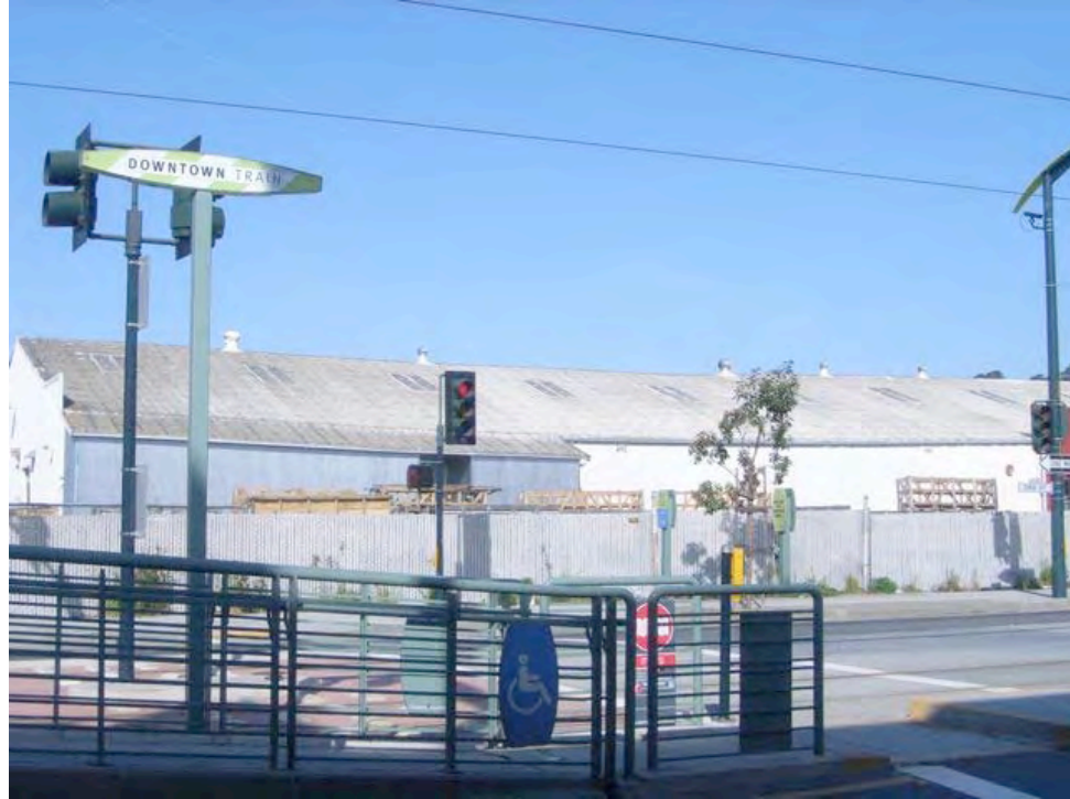
3 rd Avenue near Tulare Street: sagging roof.
