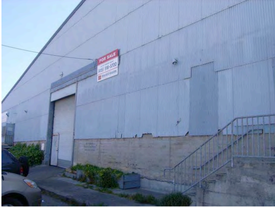
Toland Street near Galvez Avenue: deteriorated siding, dilapidation, cracked foundation.
