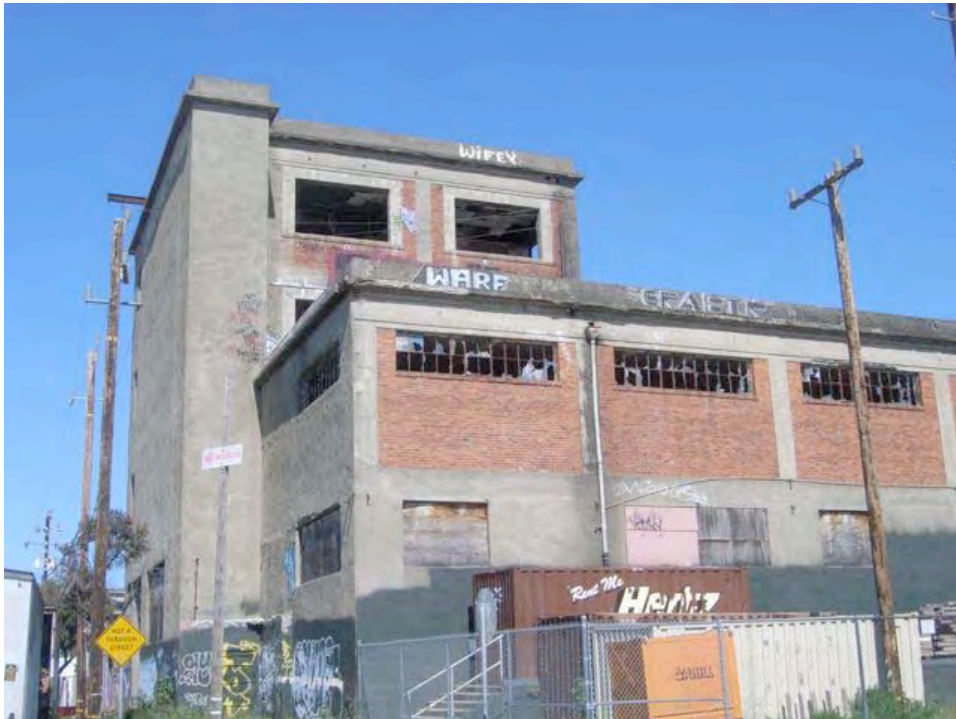
Davidson Avenue near Rankin Street: vacant and severely dilapidated industrial building, broken and boarded windows, graffiti, unreinforced masonry.
