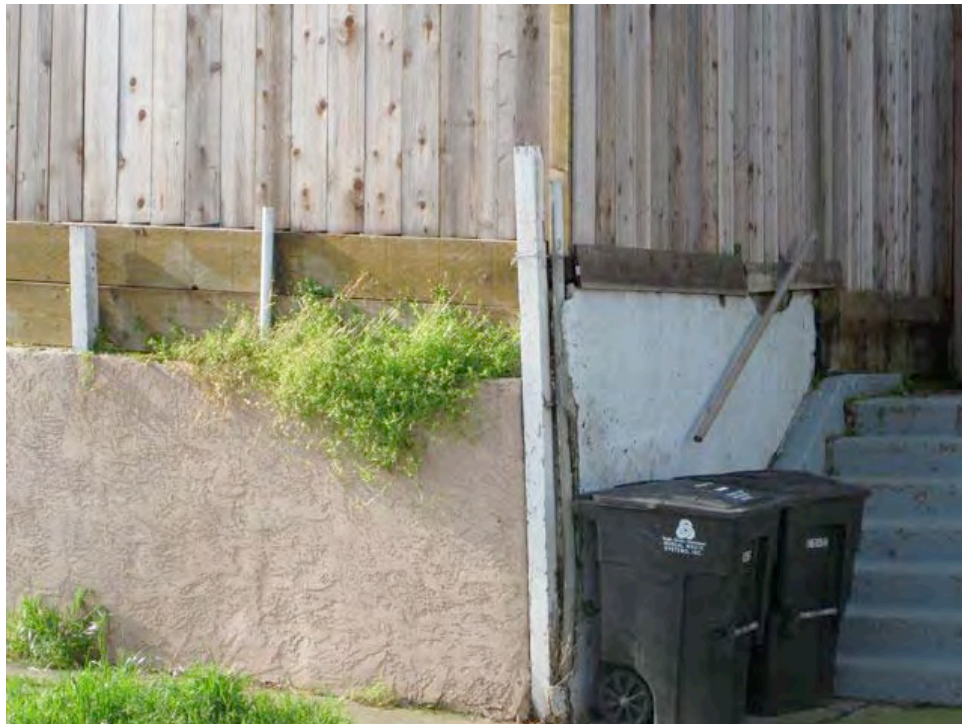
Key Avenue near 3 rd Street (close up of above): cracked retaining wall, overgrown landscaping, informal and substandard construction.
