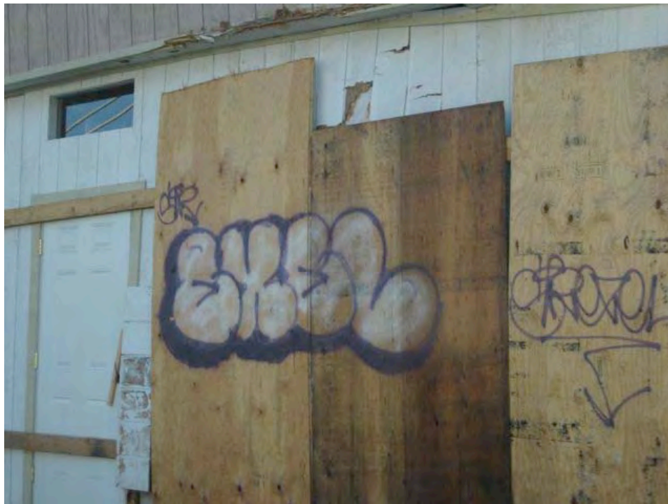
3rd Street near Palou Avenue (close up of above): boarded windows, graffiti, deteriorating siding.
